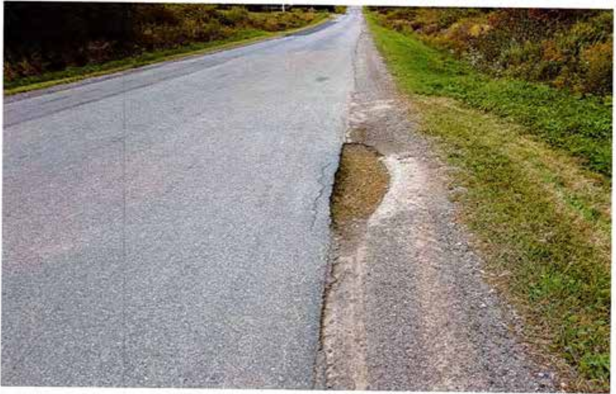
Bray Road North edge and shoulder near 2407
