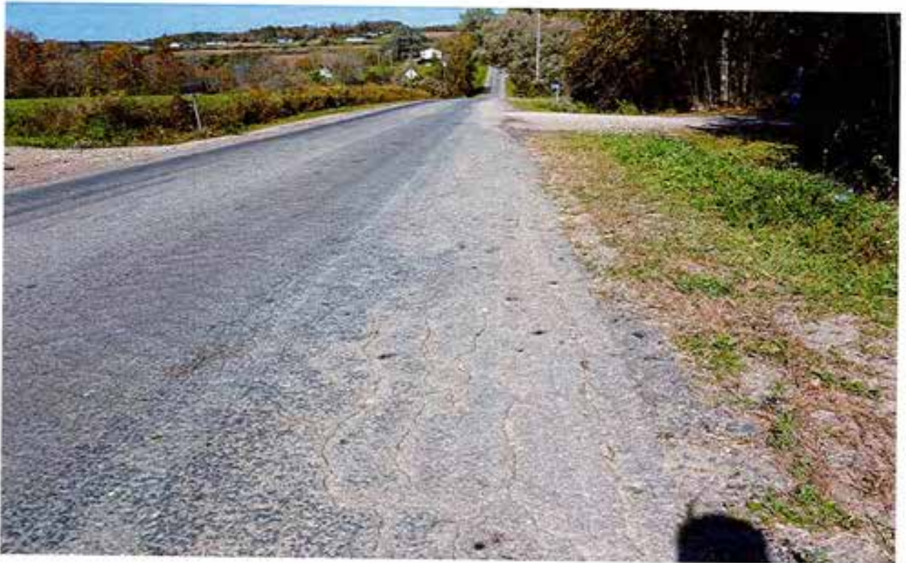
Sandbank Road East and West edge / shoulder near 10238
