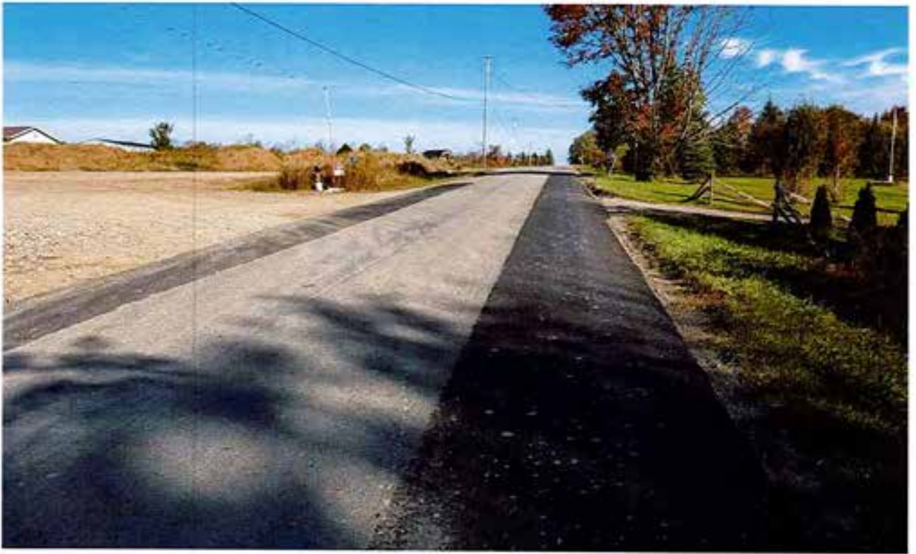
North Road North edge and shoulder near 11614 (REPAIRED)
