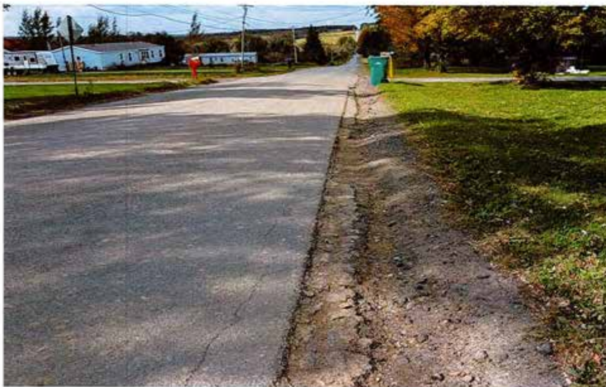
Bray Road North edge and shoulder near 2231
