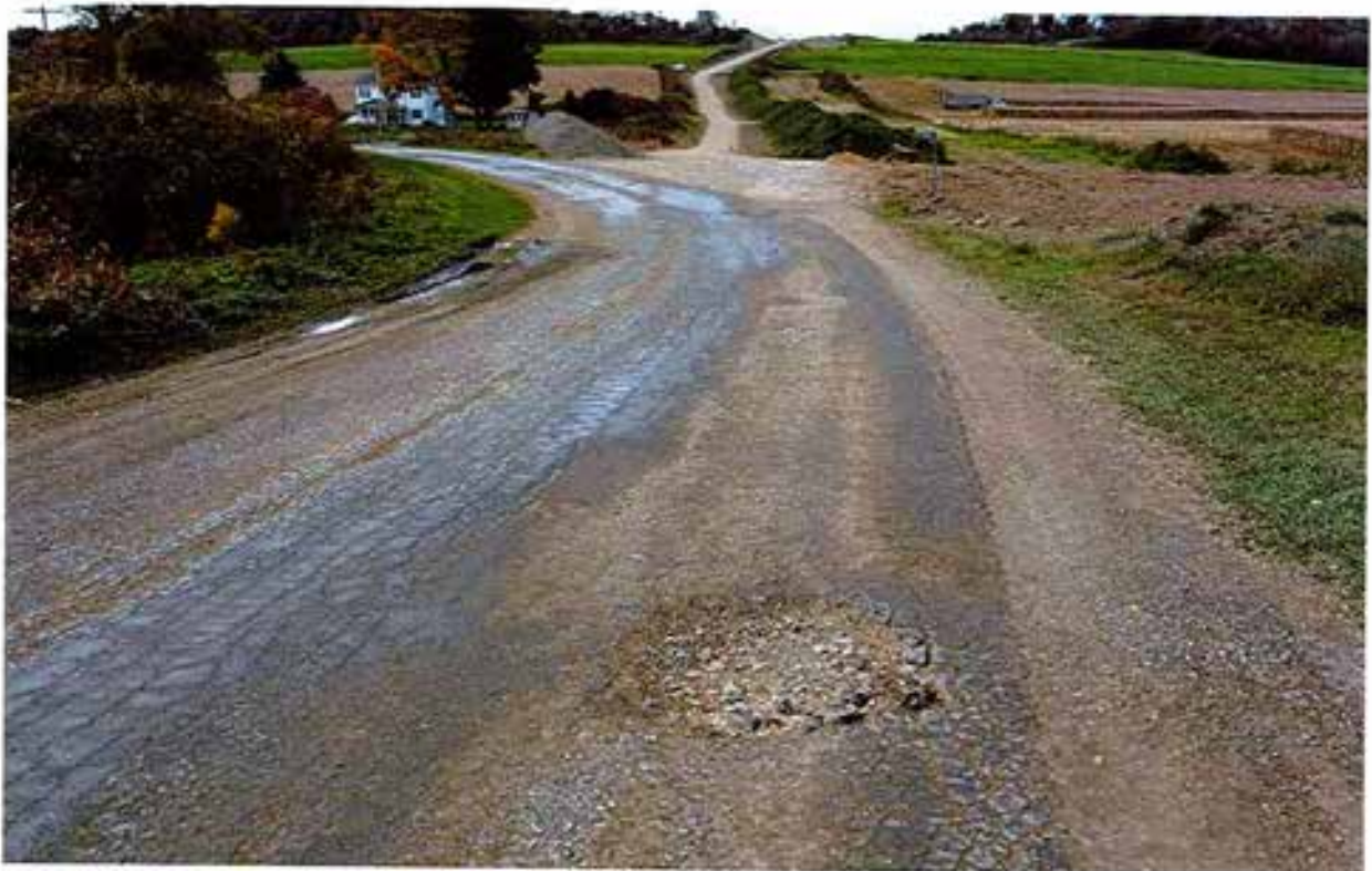
Strong Road deficiencies
