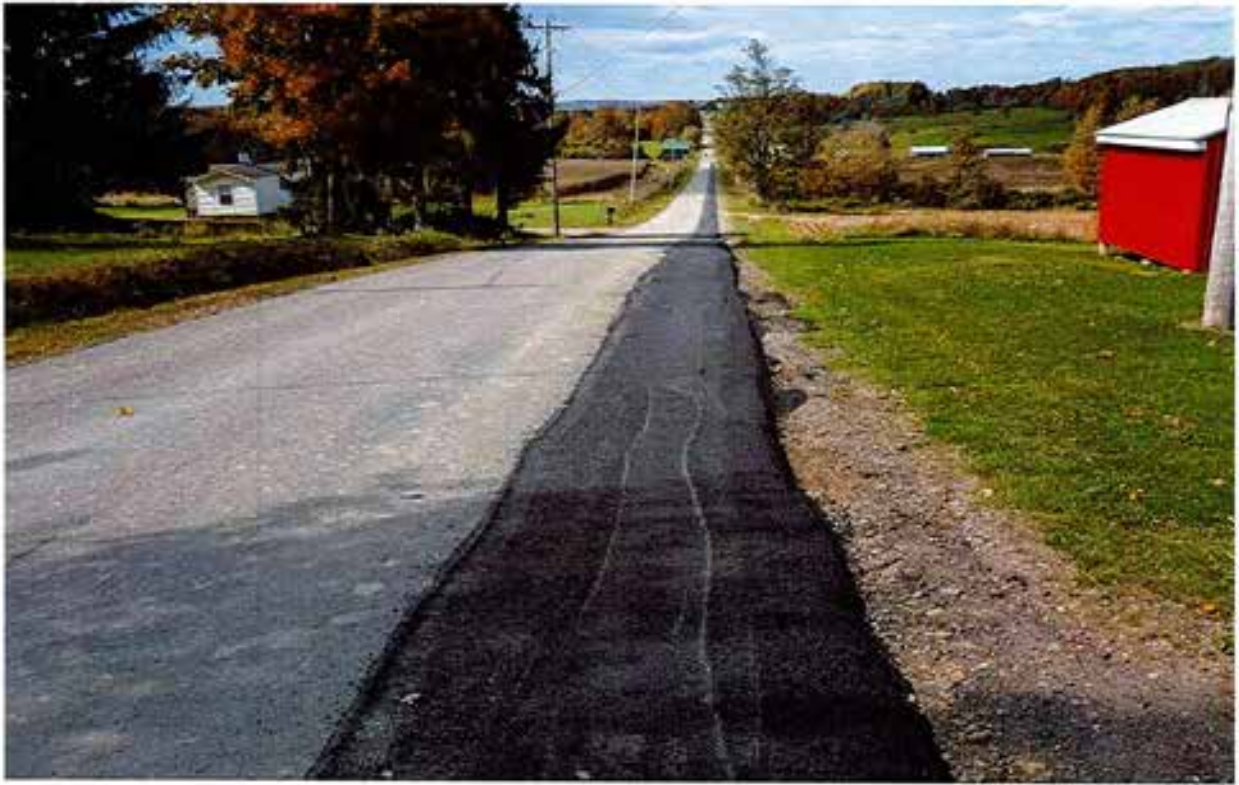
Fisher Blake Road edge and shoulder near 2177 (REPAIRED)
