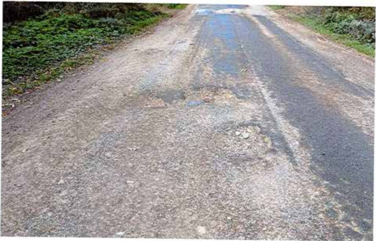
Strong Road deficiencies
