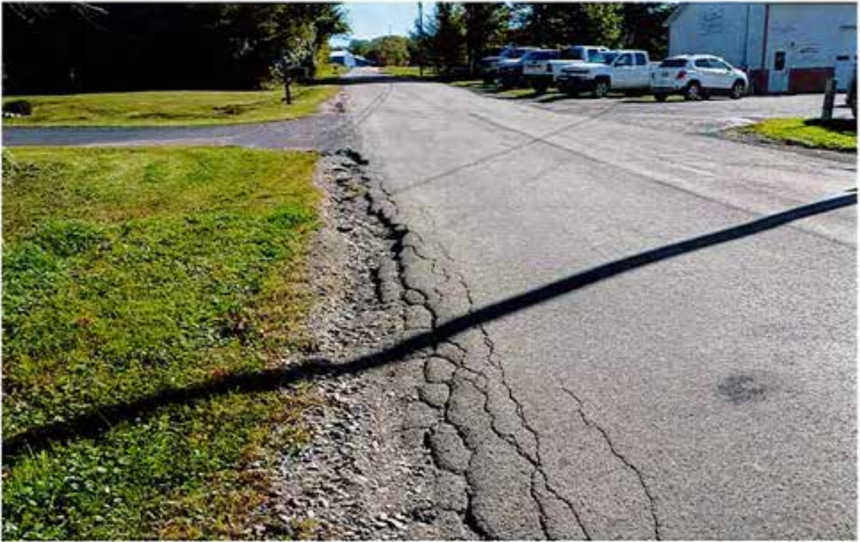
Eagle Street East and West side lane and edge deterioration near 1244
