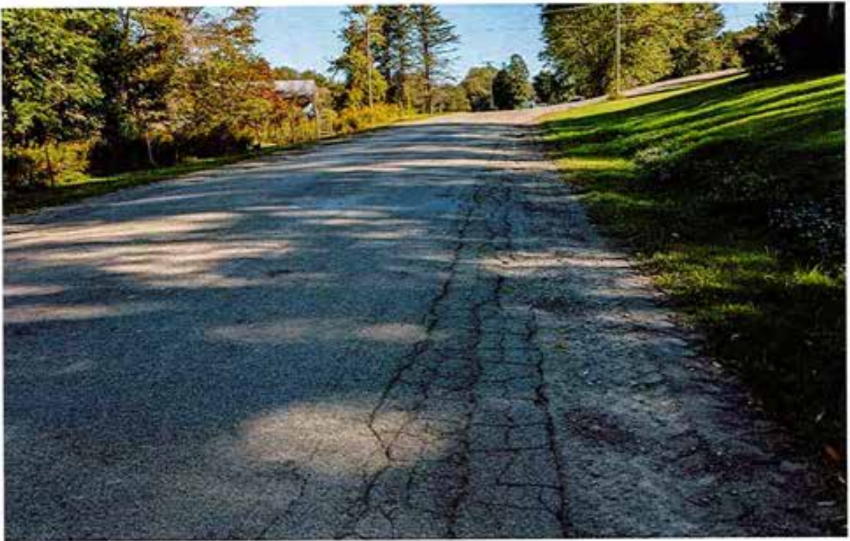
Eagle Street East edge deterioration near Hughes
