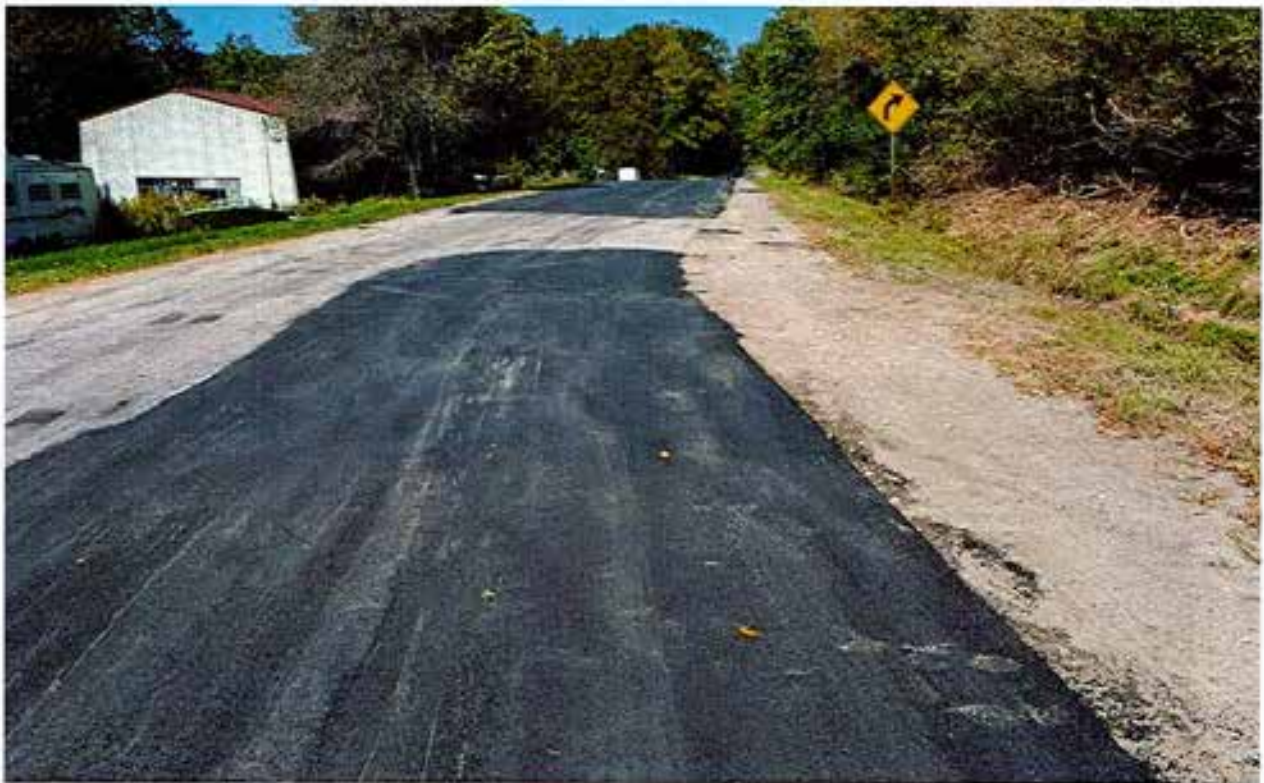
Osmun Rd Edge and shoulder deterioration near Zimmer (REPAIRED)
