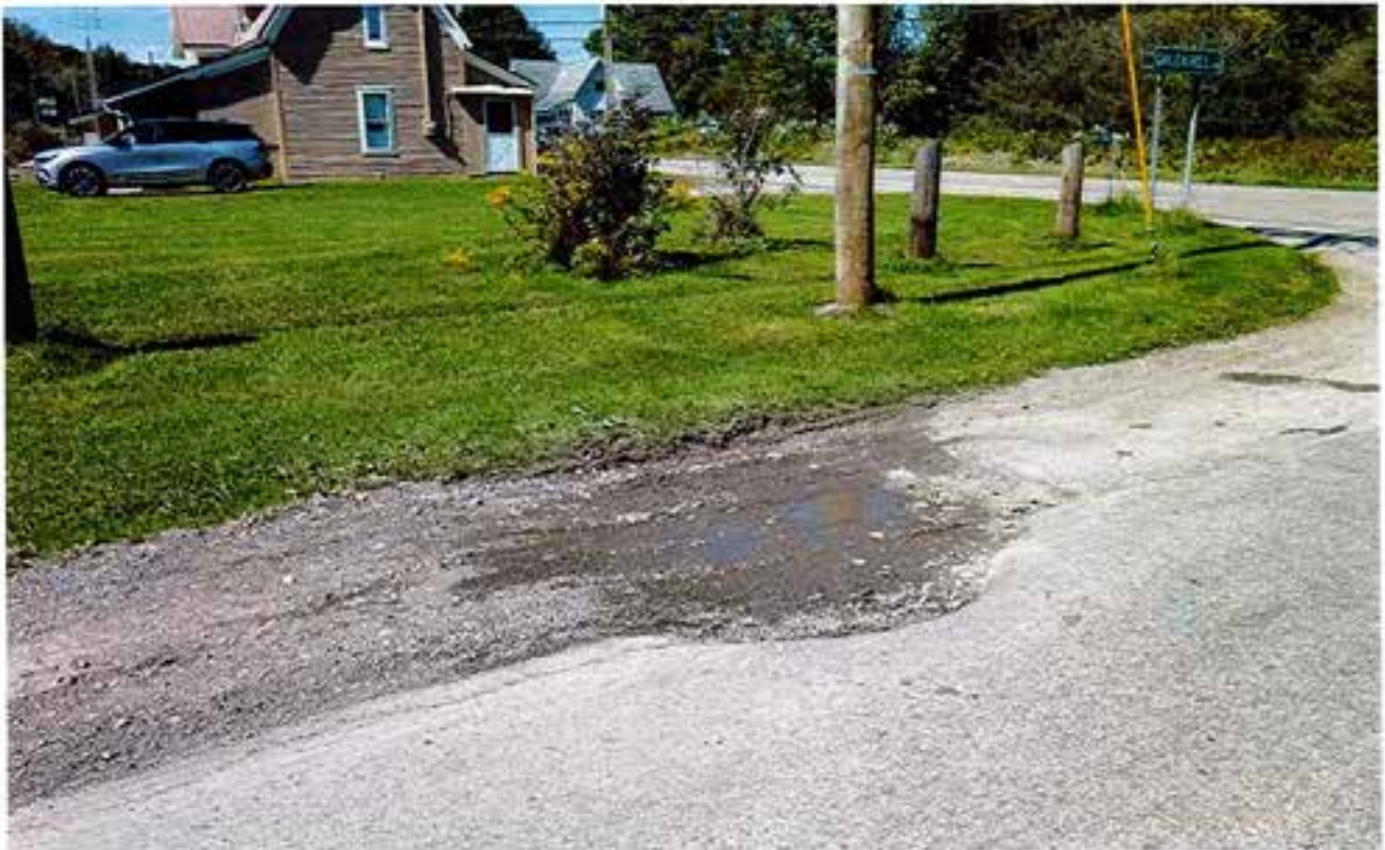
Galen Hill Rd pothole at intersection of Route 98
