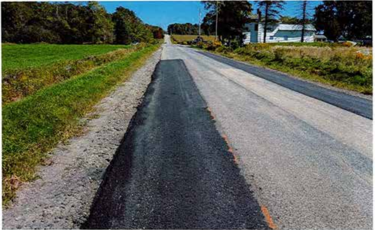
Baird Rd North shoulder deterioration East and West of 379 (REPAIRED)
