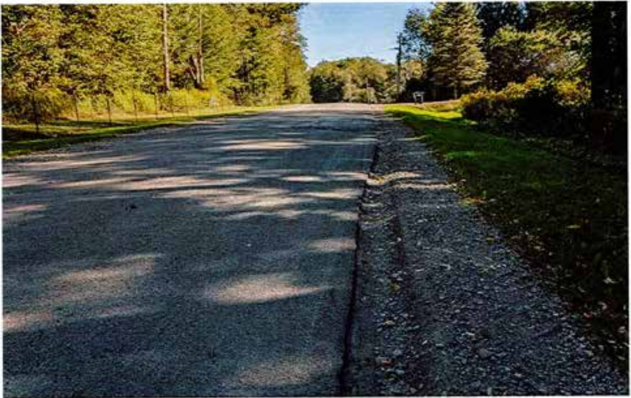
Eagle Street lane and shoulder deterioration near 1111
