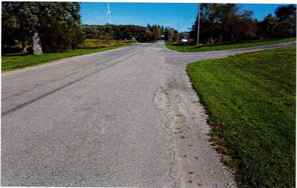
Eagle Street East edge and shoulder deterioration near 757
