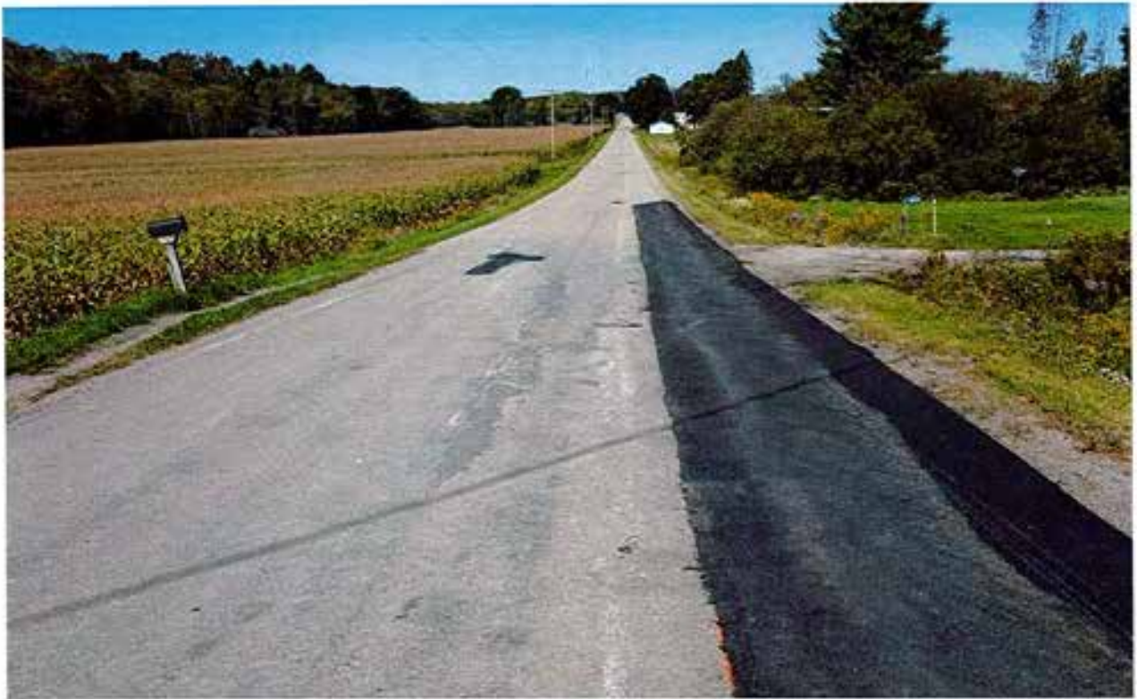
Osmun Road lane deterioration near 10674
