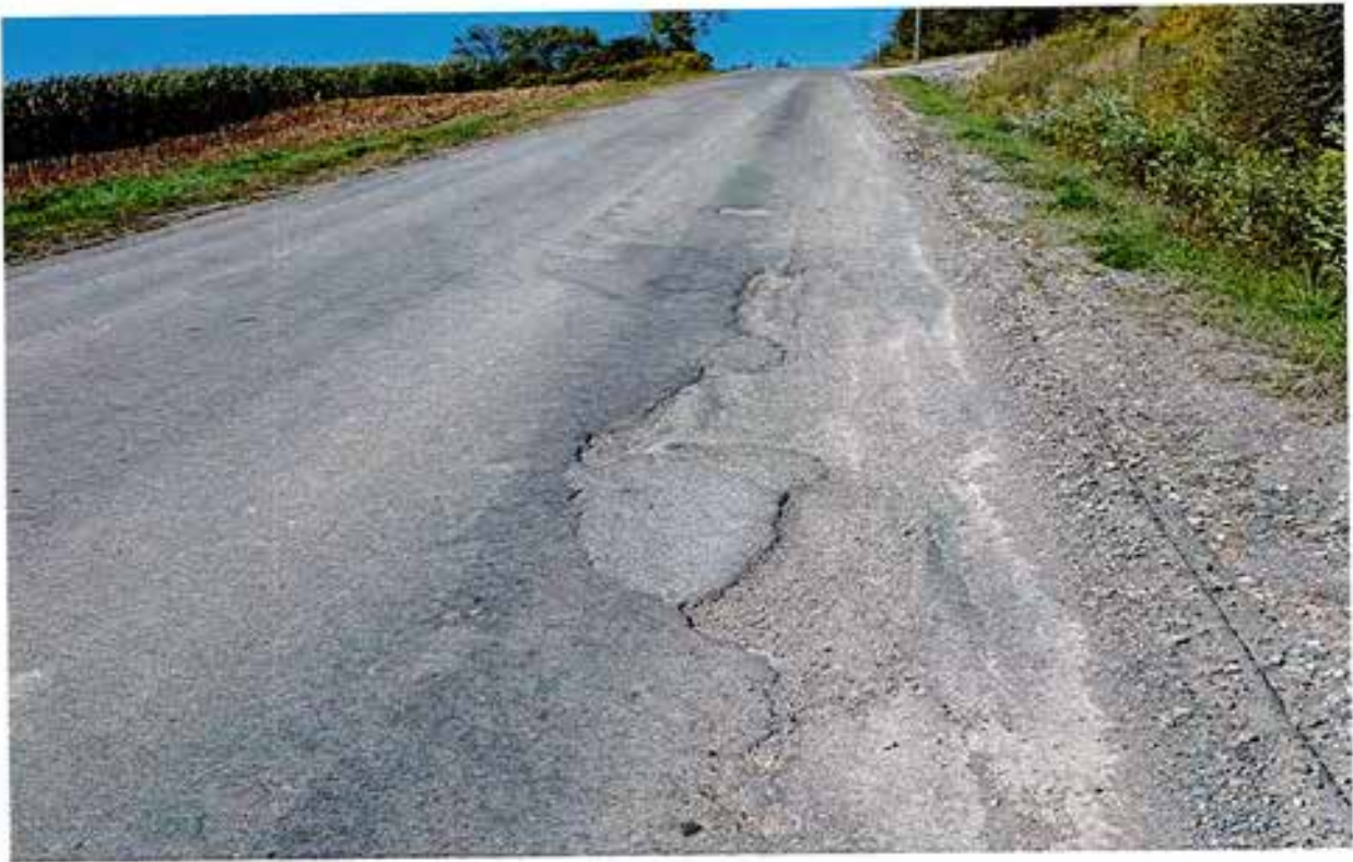
Bray Road lane deterioration near 2801 (#2)
