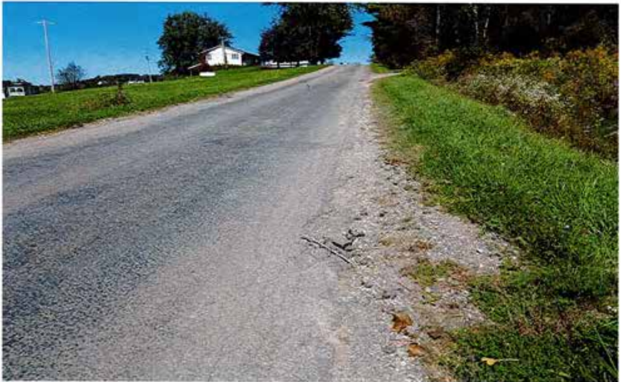
Sandbank Rd East lane and edge deterioration South of 10317
