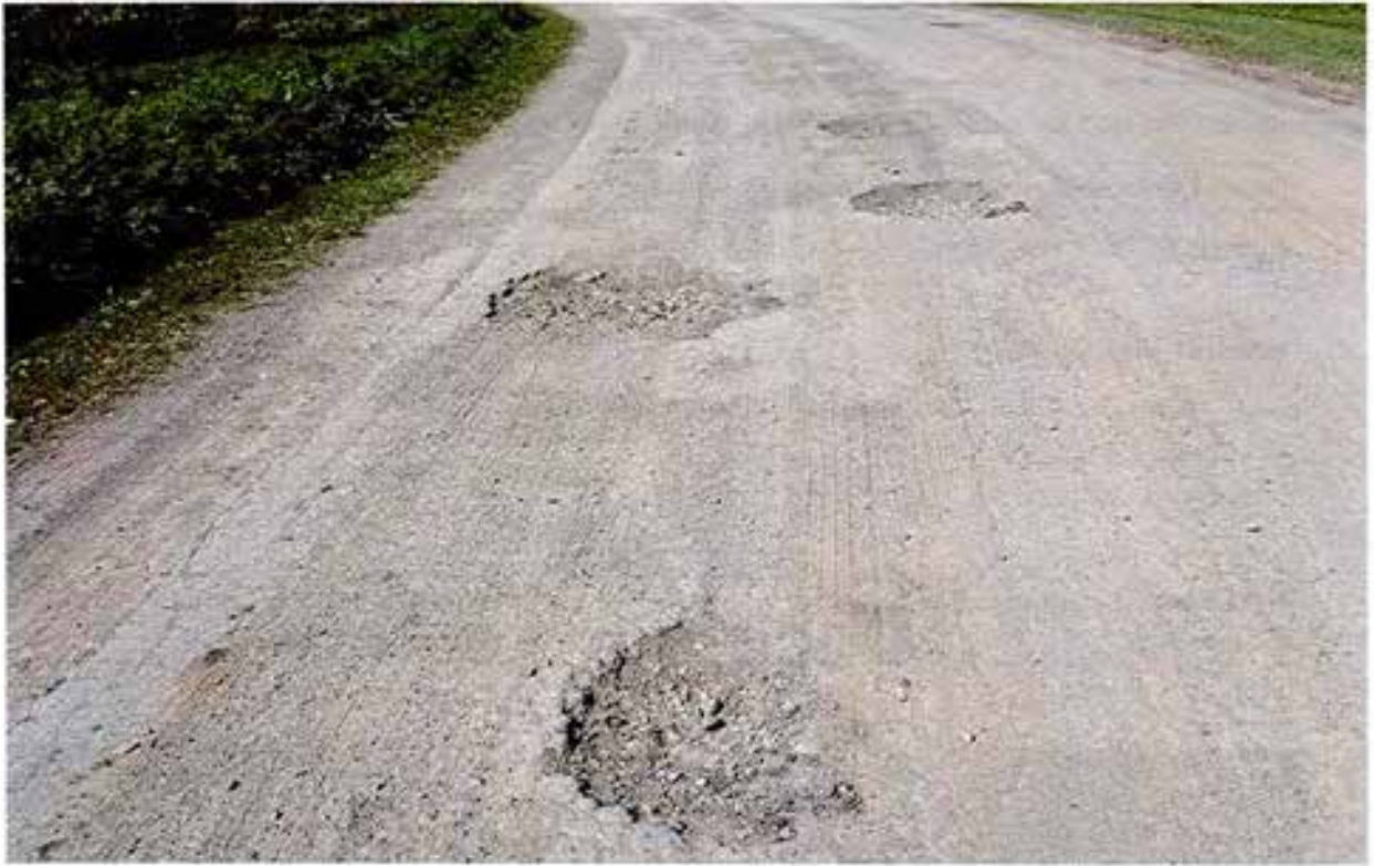
Strong Rd potholes
