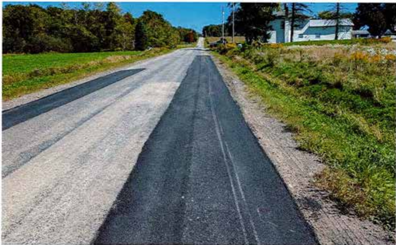
Baird Rd South shoulder deterioration East and West of 379 (REPAIRED)
