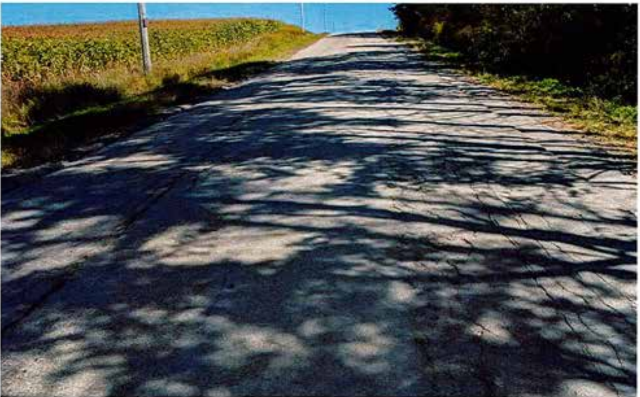
Baird Road lane deterioration from 253 to 187
