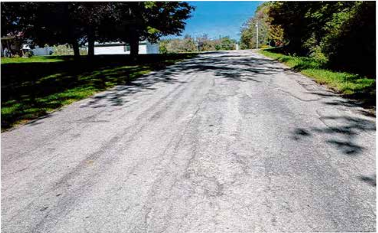
Sandbank Rd lane deterioration near 10317
