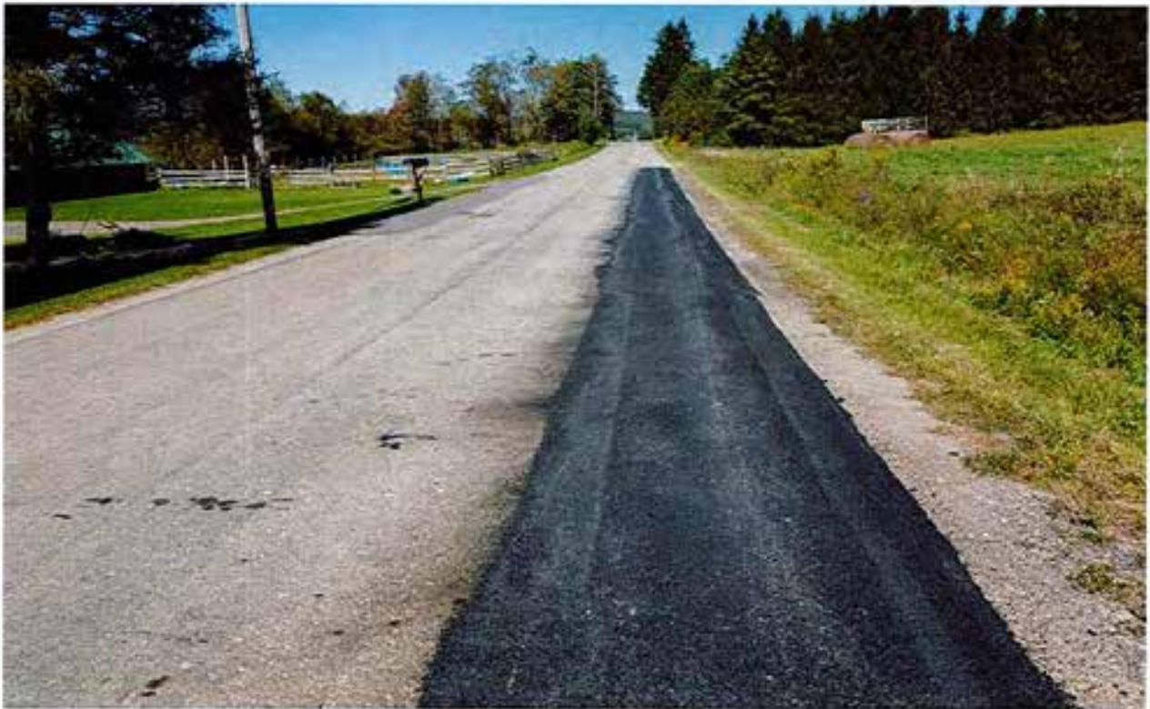
Osmun Road East edge and shoulder deterioration near 10571 (REPAIRED)
