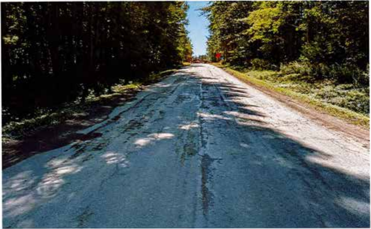
Galen Hill Road lane deterioration from Phillippi Rd to 10553
