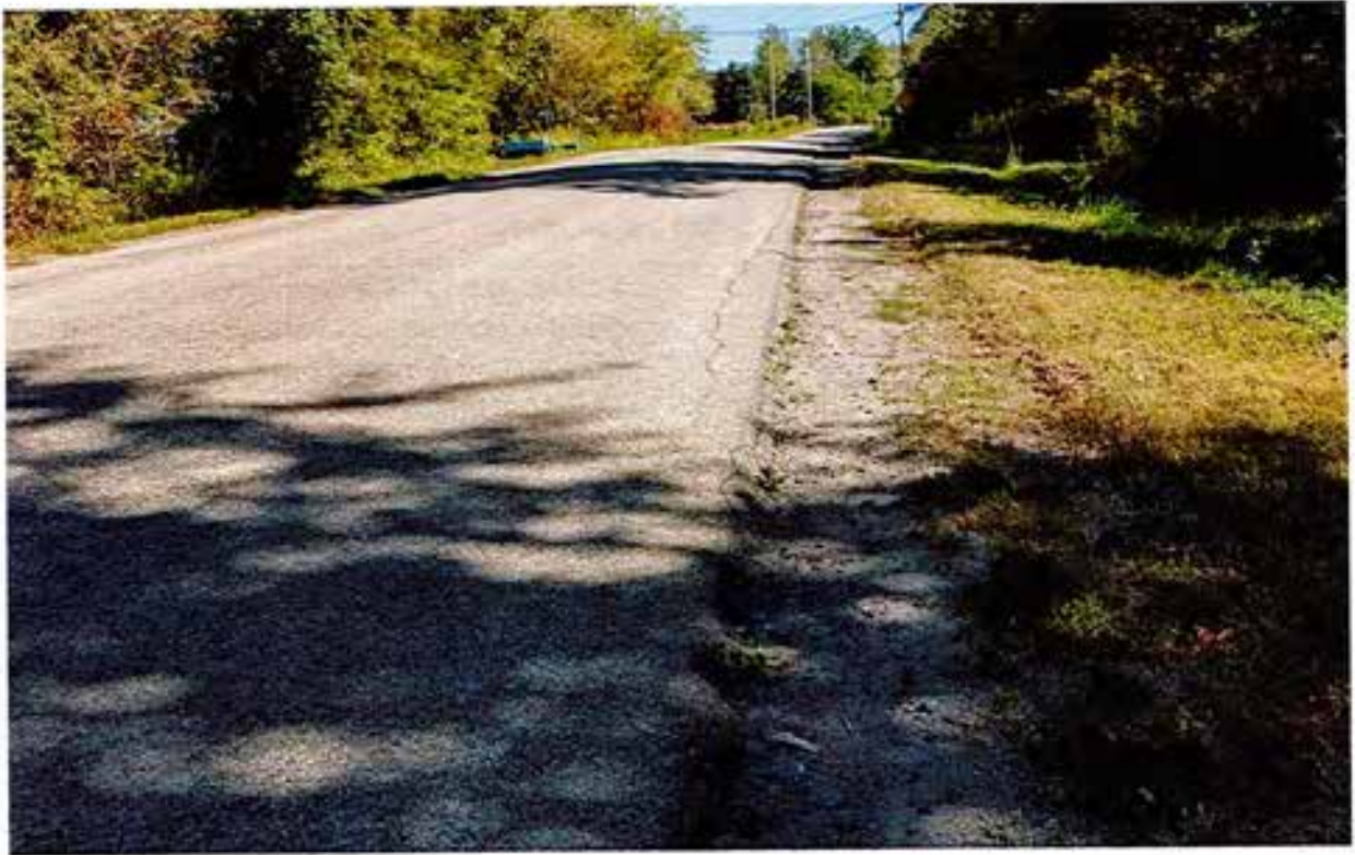
Edmunds Road South edge and shoulder deterioration 1940 to 1850
