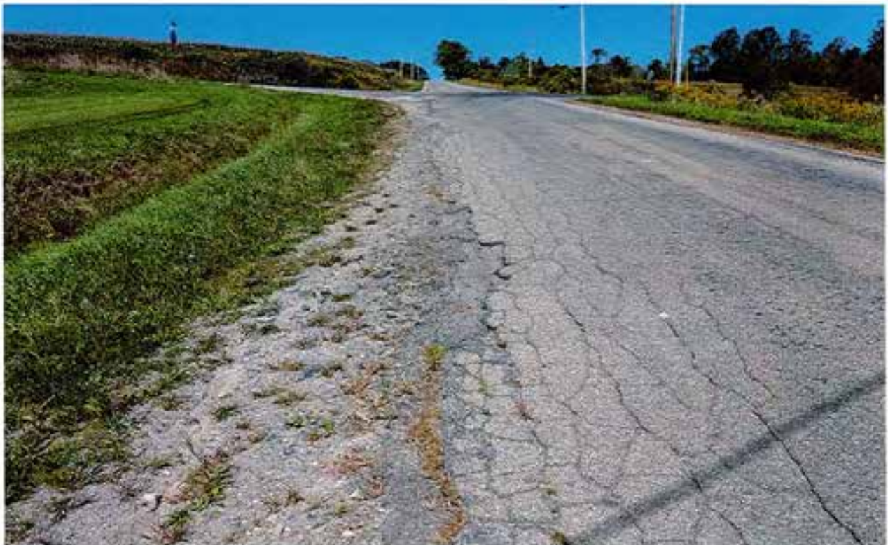
Sandbank Road (East and West) edge and shoulder deteriorating near intersection with Cross Road
