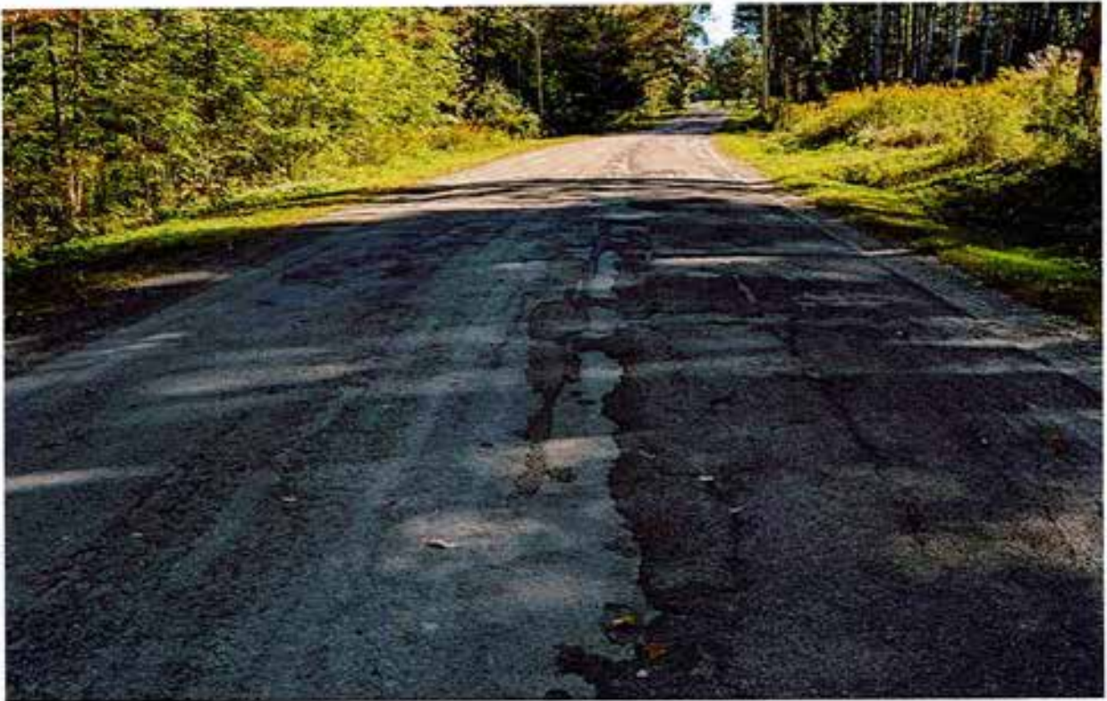
Eagle Street lane deterioration near 915
