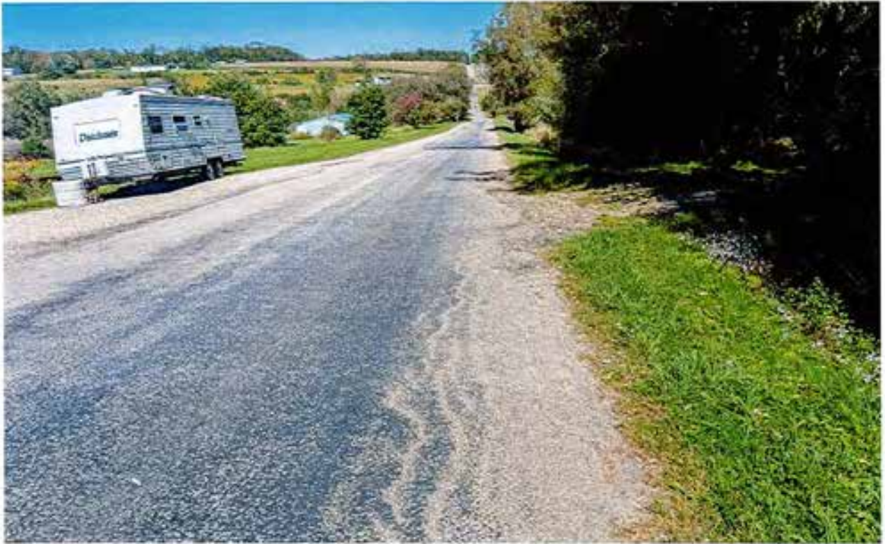
Sandbank Rd East and West side shoulder deterioration near 10442
