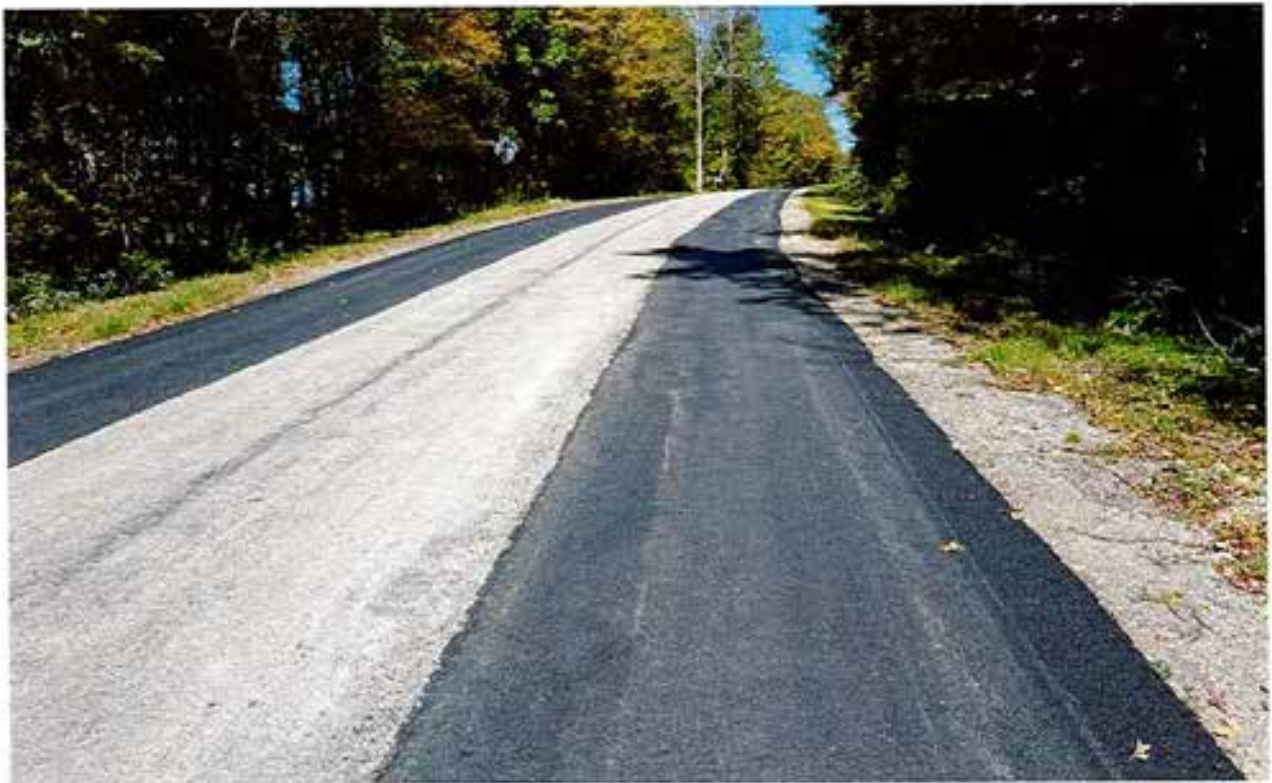
Osmun Road lane deterioration South of 10200 (REPAIRED)
