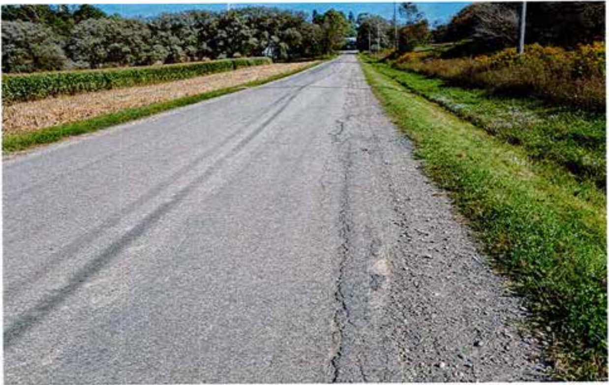
Eagle Street lane and edge deterioration North of 757
