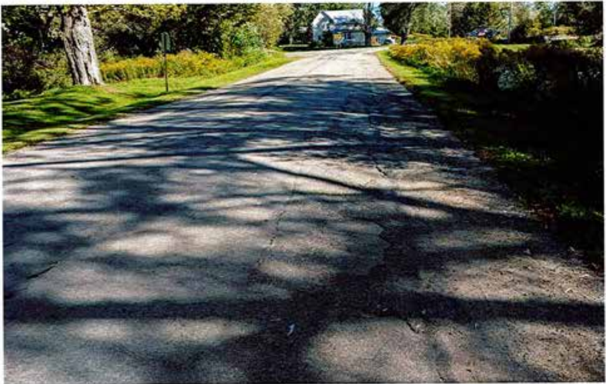
Eagle Street East lane deterioration near 708
