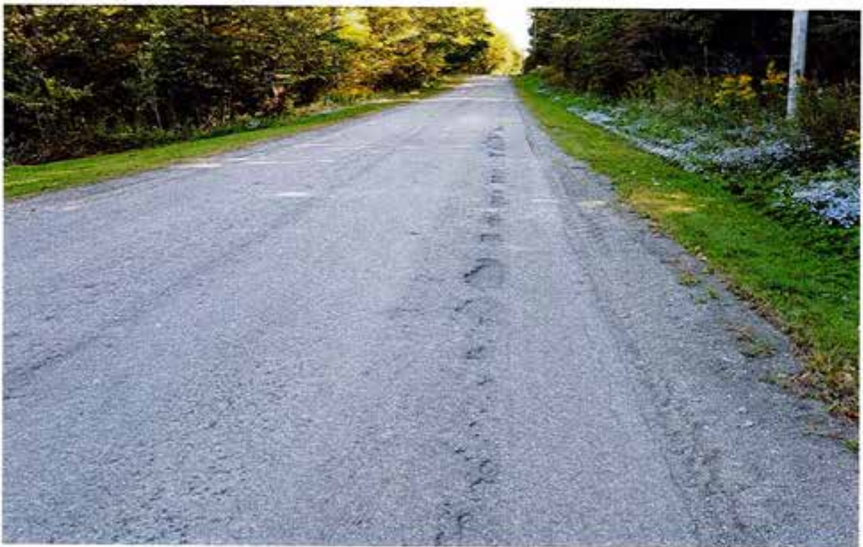
Eagle Street lane deterioration near 1000
