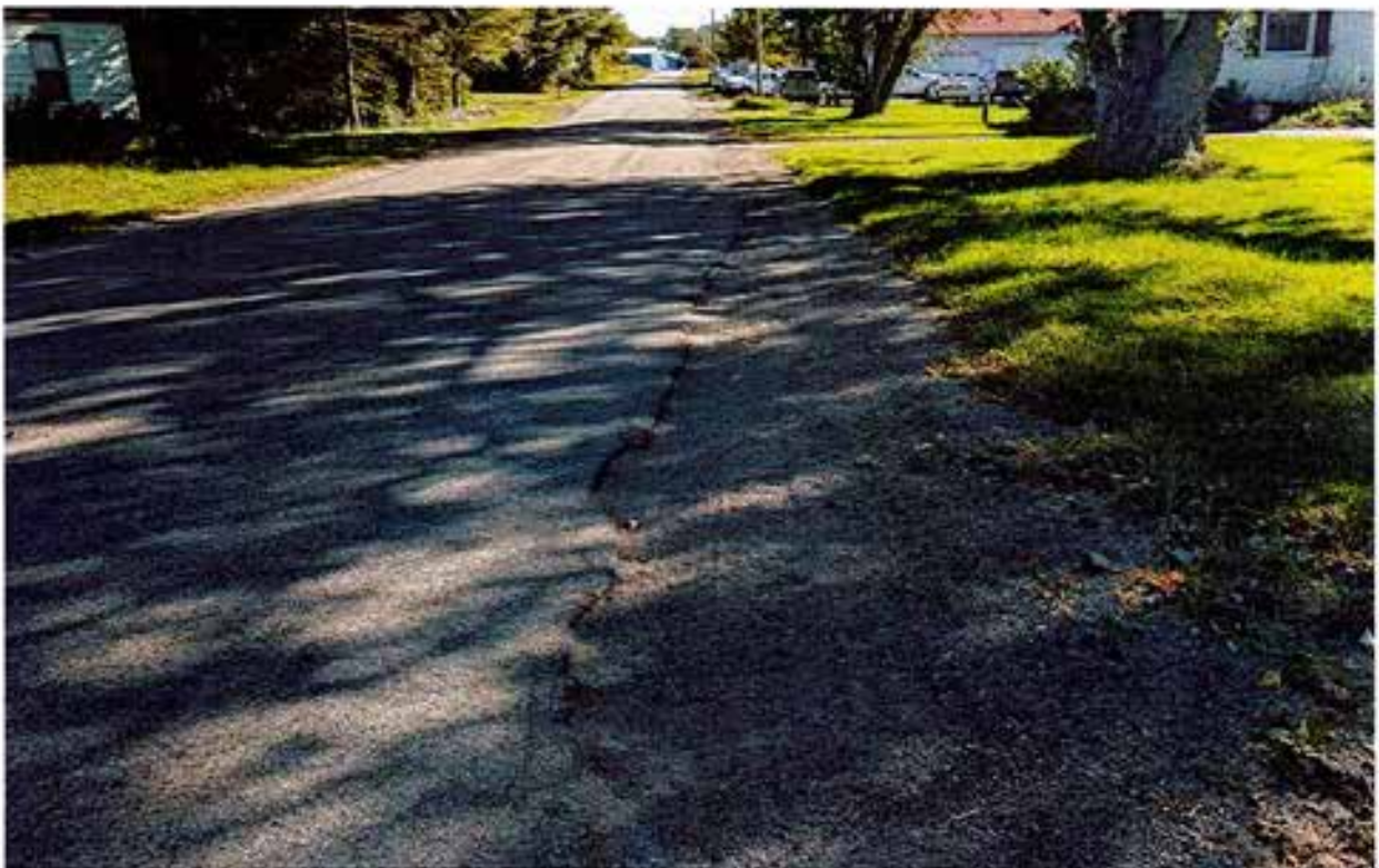
Eagle Street lane and edge deterioration near 1253
