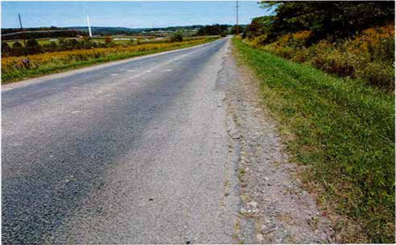
Sandbank Rd East and West edge deterioration North and South of 10157 to +/- 10220
