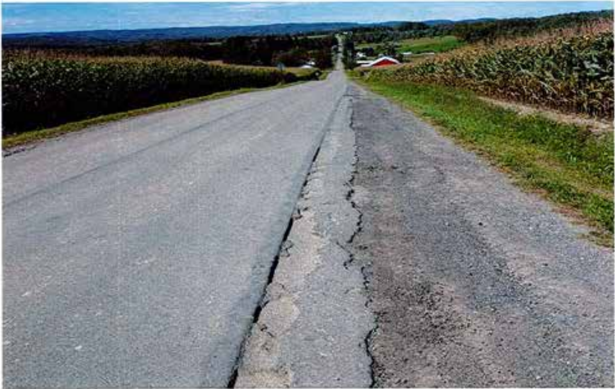
Fisher Blake Road North edge and shoulder deterioration near intersection with Brown Schoolhouse Road
