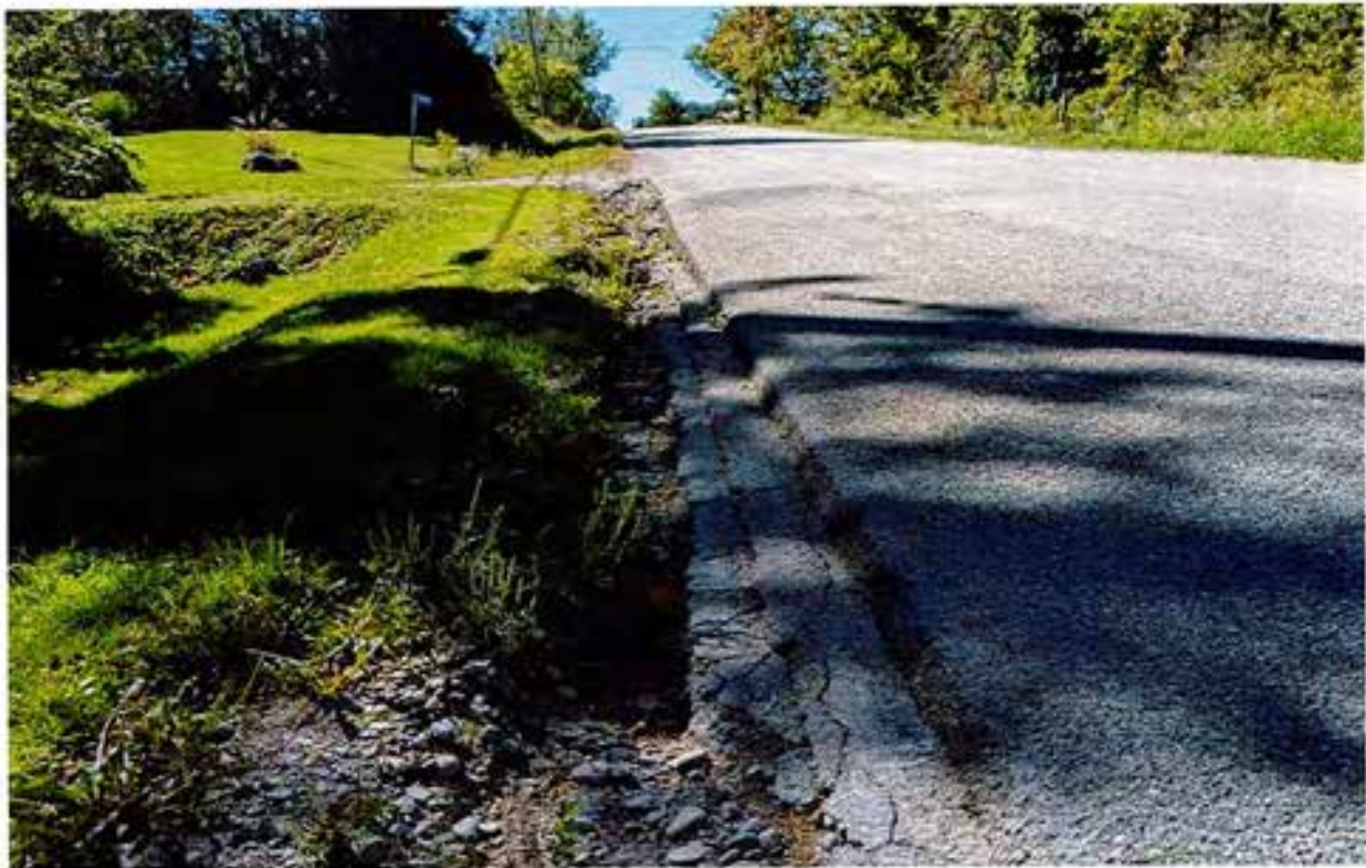
Brown Schoolhouse Road East edge and shoulder deterioration from 11754 to 11740
