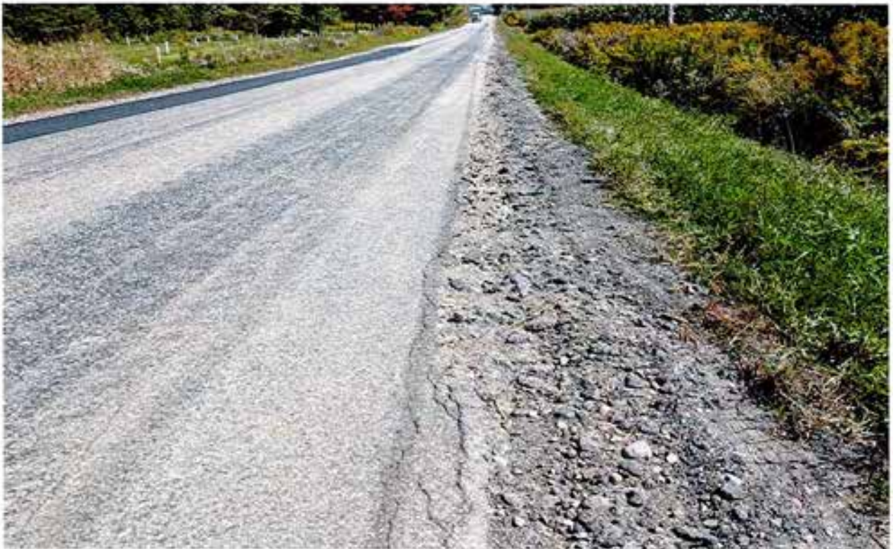
Baird Road South edge deterioration from +/- 379 to +/- 253
