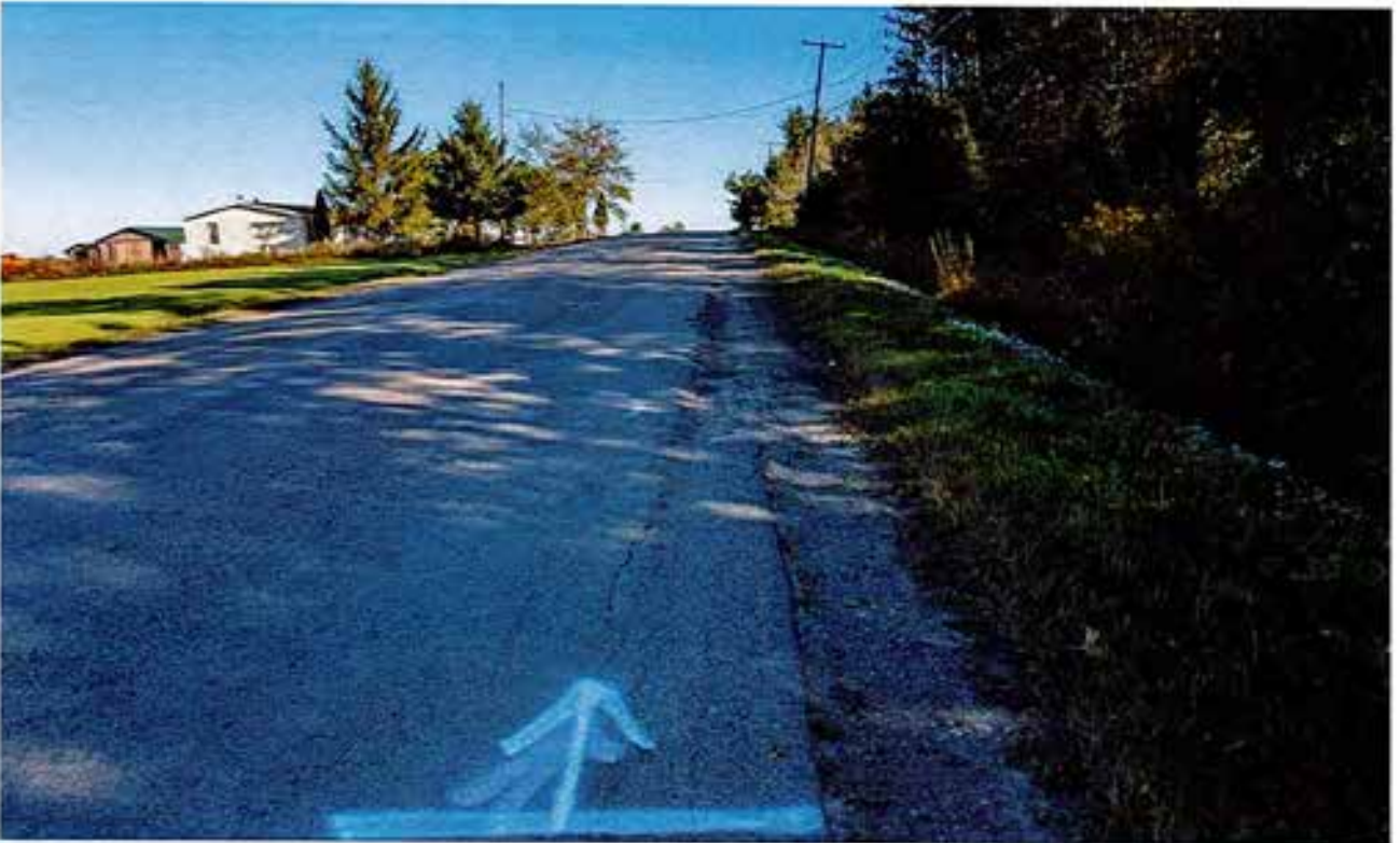
North Road lane and edge deteriorating with South of 11875
