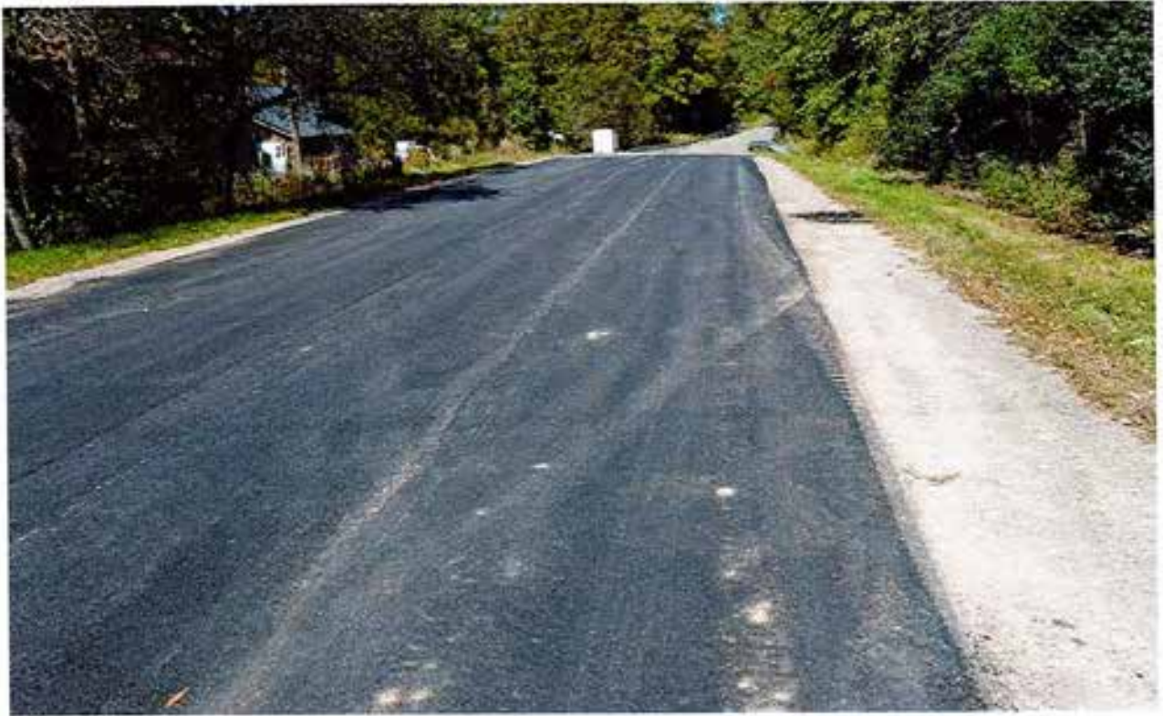
Osmun Rd lane deterioration near Zimmer (REPAIRED)
