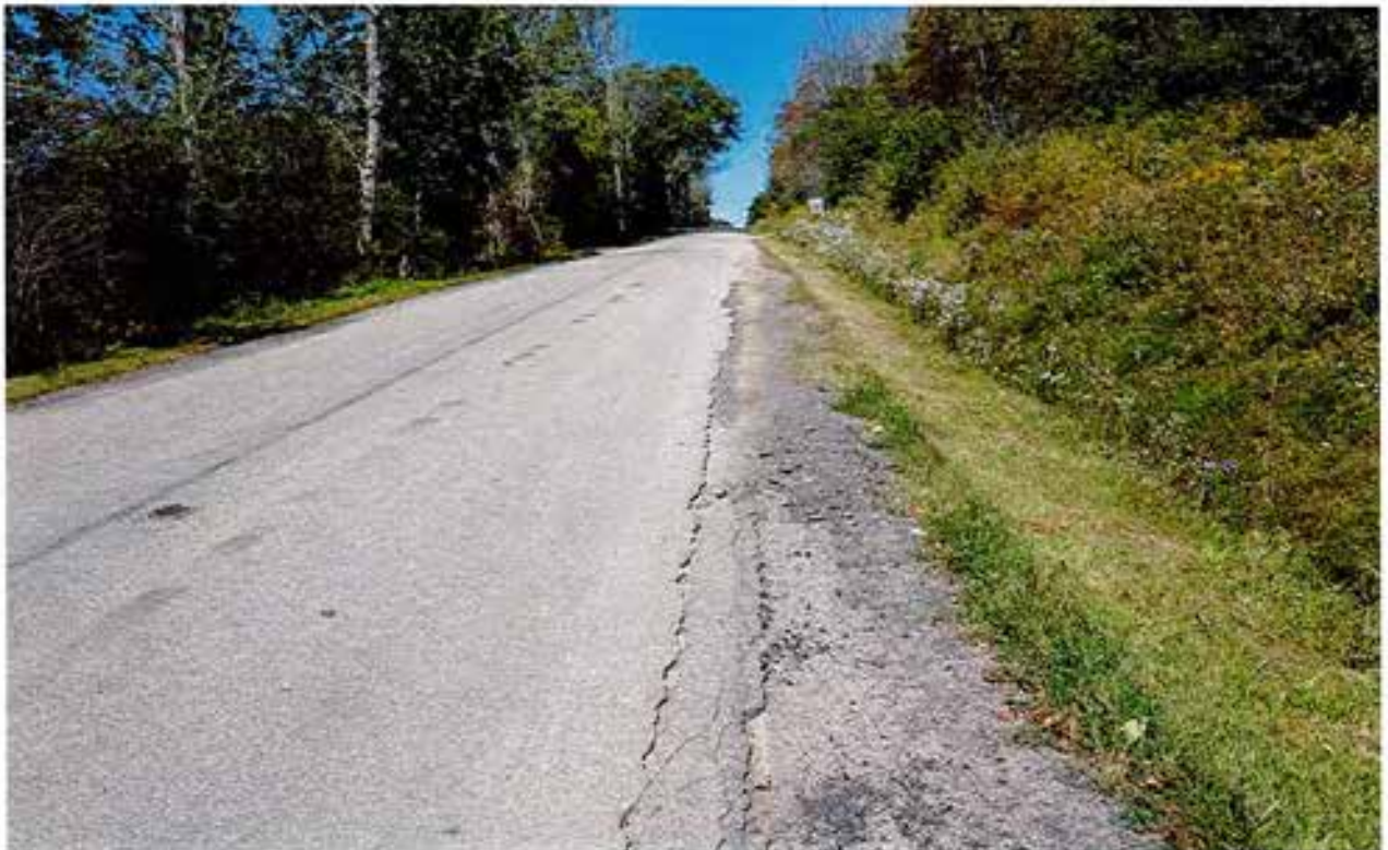
Osmun Rd East side lane, edge, and shoulder deterioration North and South of 10410
