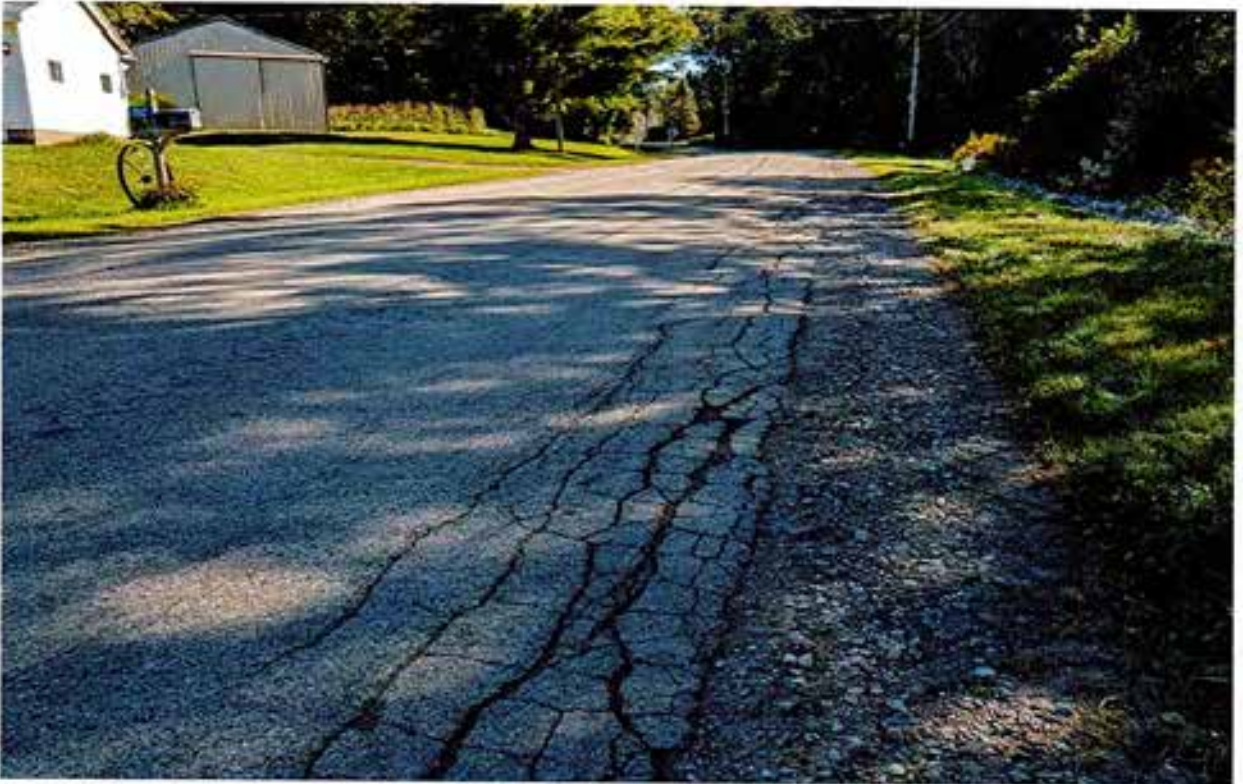
Eagle Street lane and edge deterioration near 1152
