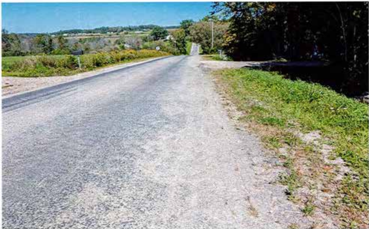
Sandbank Road East and West edge / shoulder deterioration near 10238
