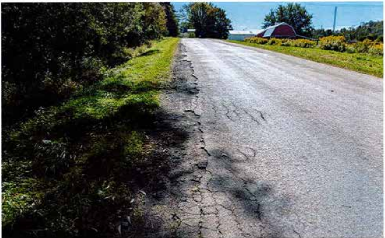
Sandbank Road East edge deterioration South of 10368
