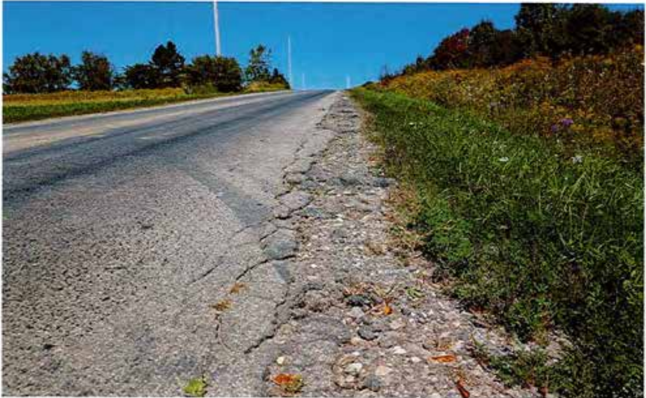
Sandbank Road East edge and shoulder deterioration near 9999
