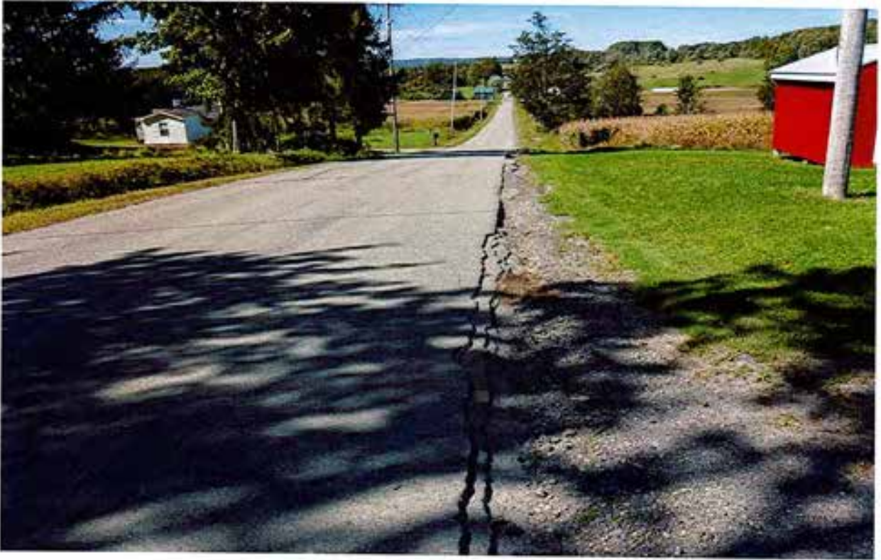
Fisher Blake Road edge and shoulder deterioration near 2177
