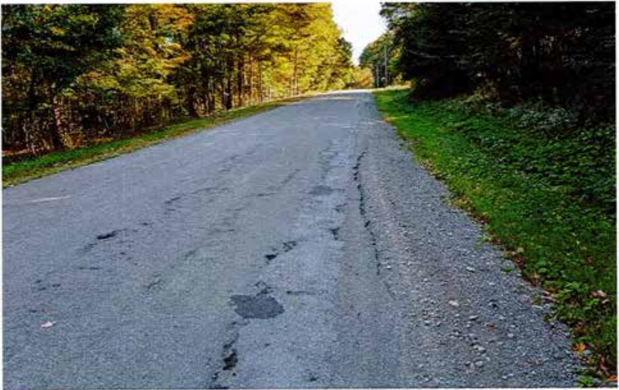
Eagle Street lane and edge deterioration near 931
