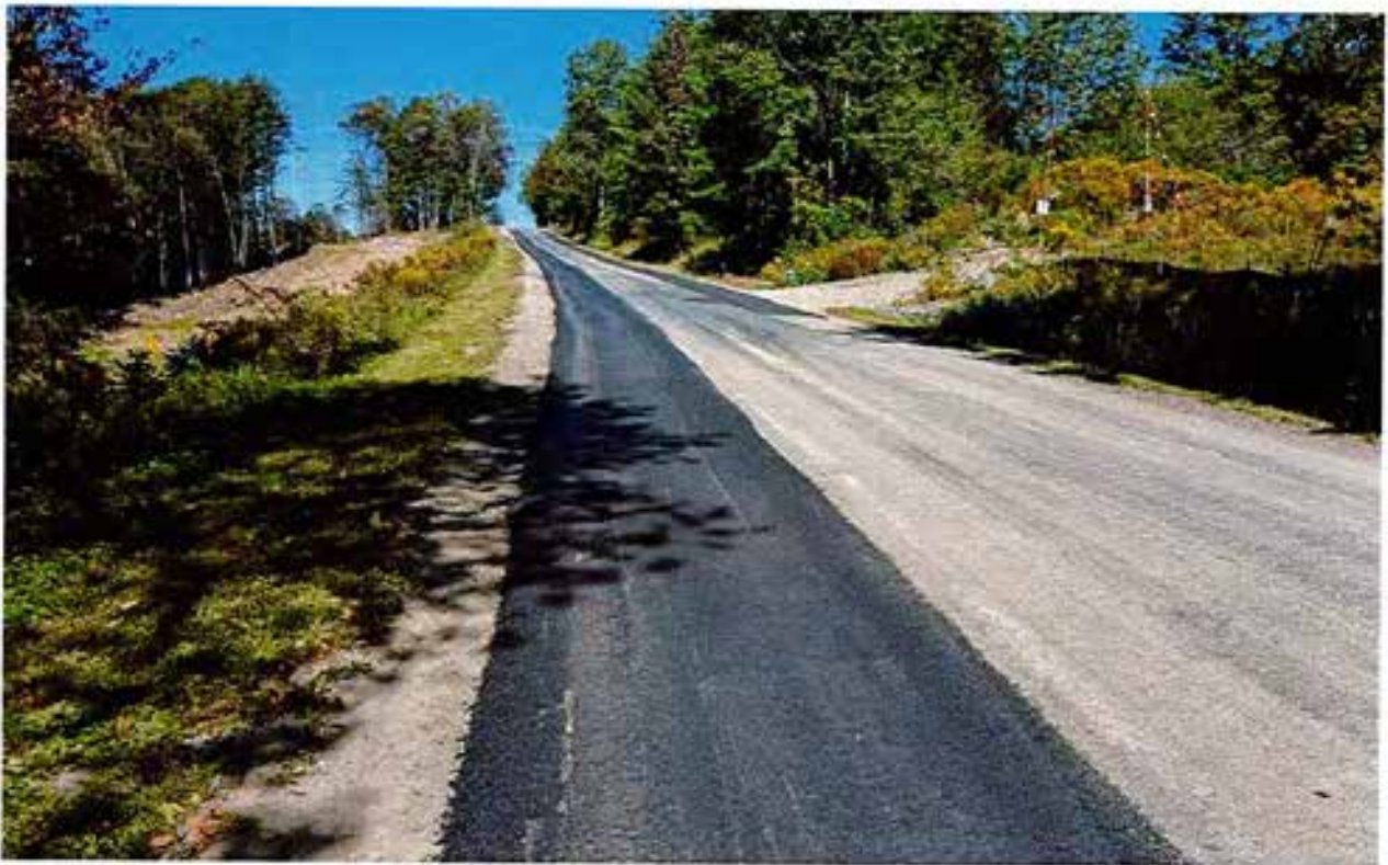
Osmun Rd lane deterioration North of 10220 near construction entrance (REPAIRED)
