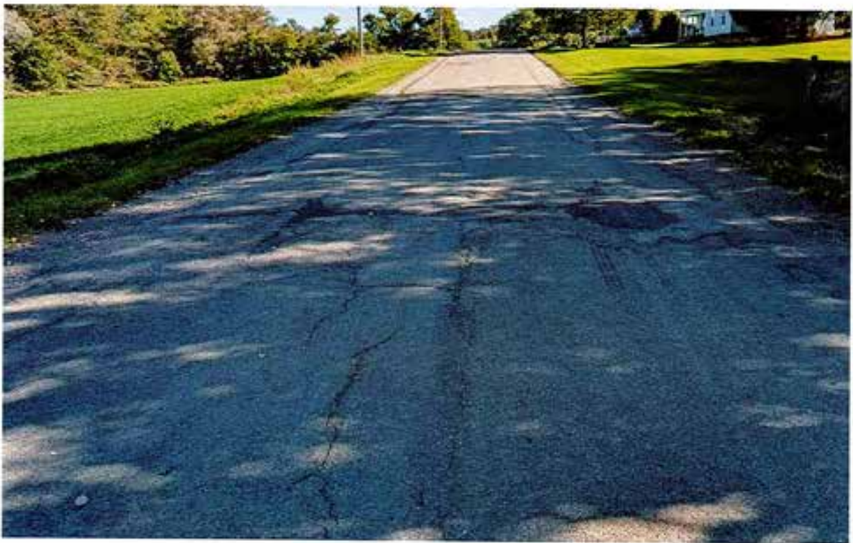
Eagle Street lane deterioration South of 849
