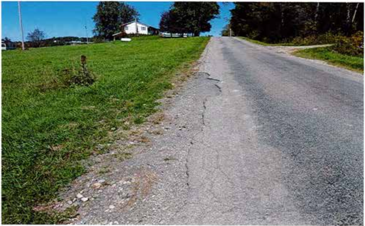
Sandbank Rd West lane and edge deterioration South of 10317
