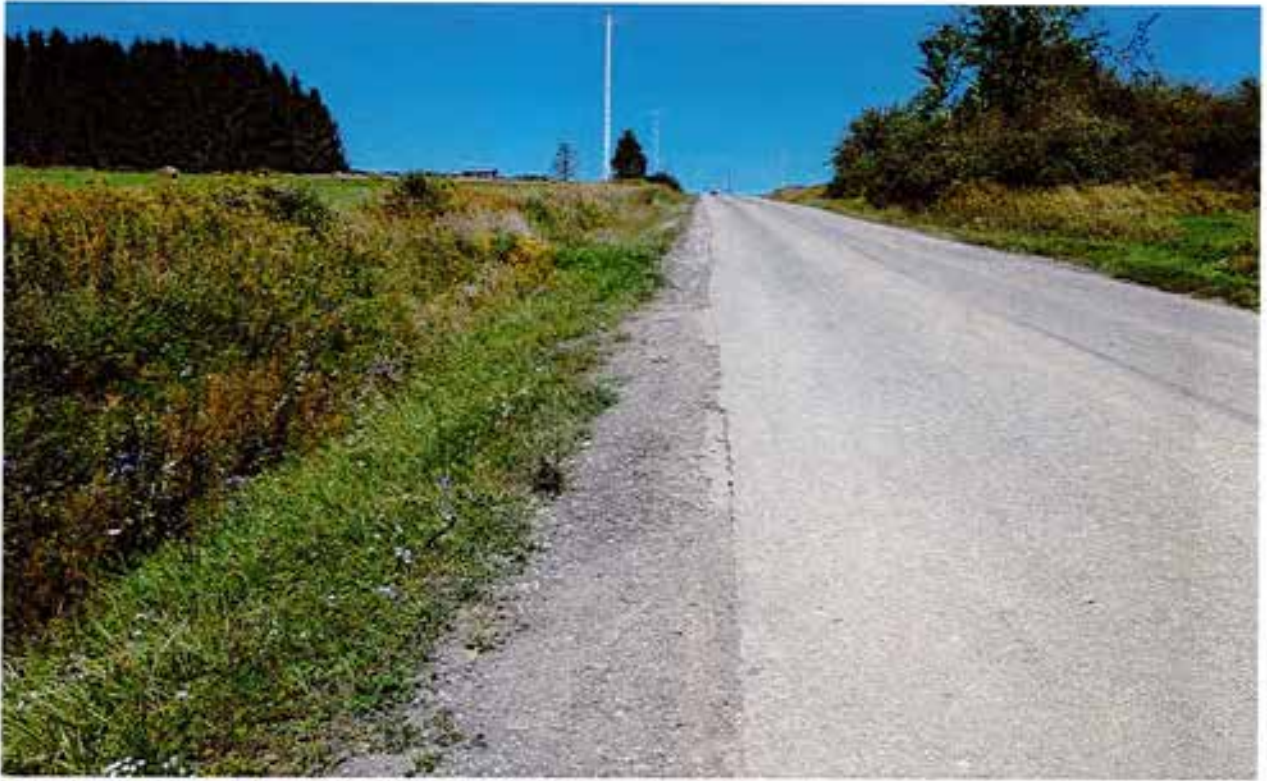
Galen Hill West edge and shoulder deterioration North of 10075
