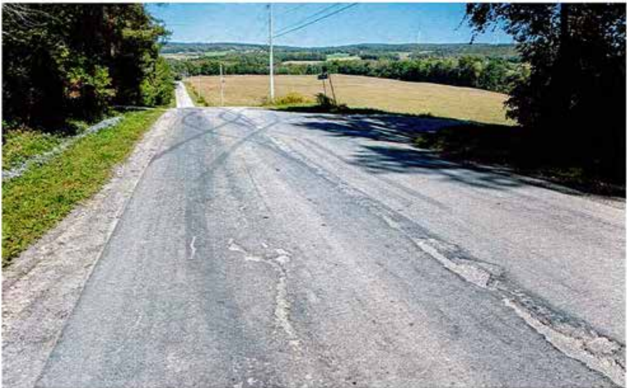
Galen Hill Road intersection with Phillippi Rd lane deterioration
