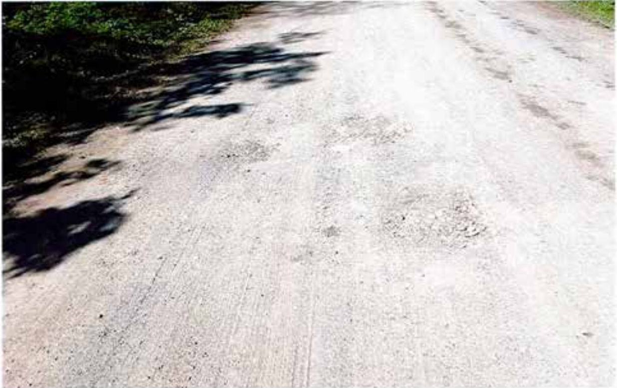
Strong Road potholes
