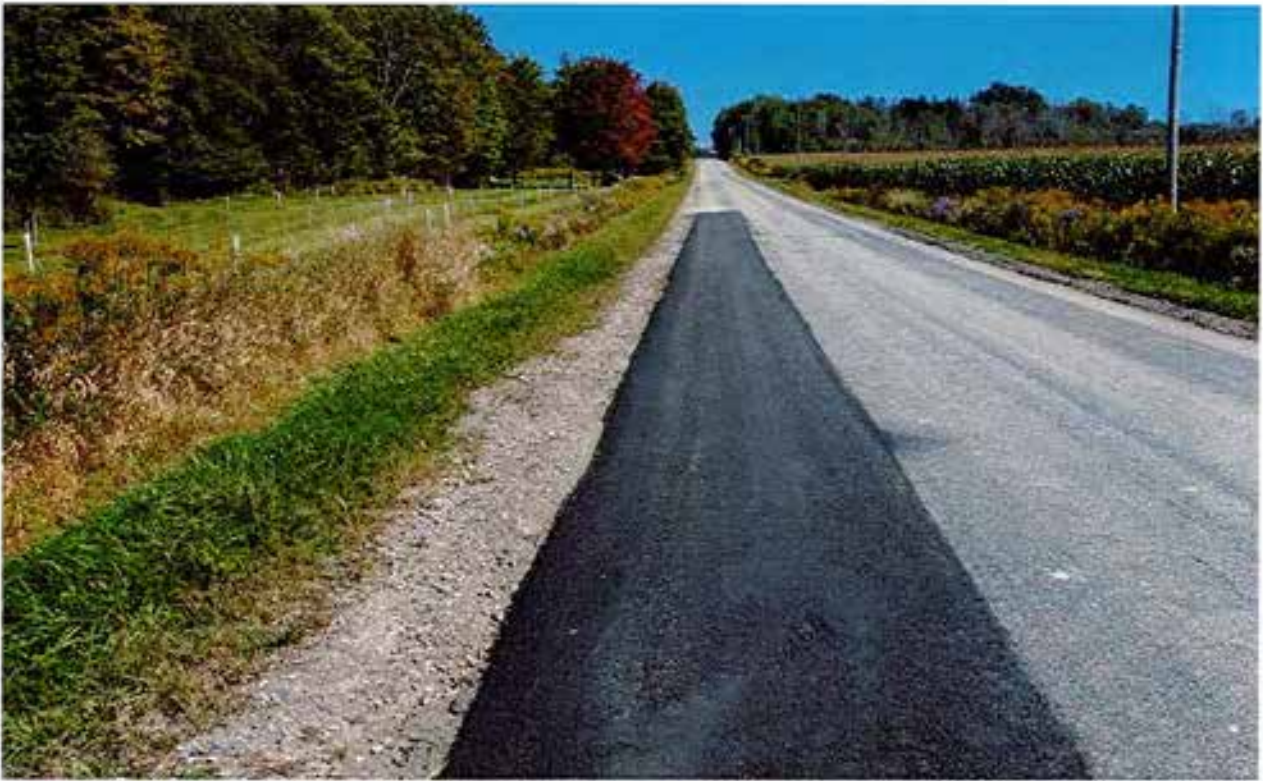
Baird Road North edge deterioration from +/- 379 to +/- 253 (REPAIRED)
