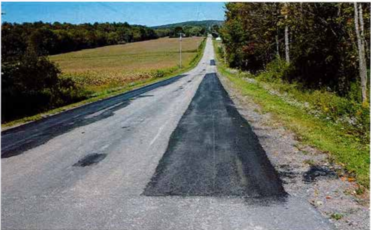
Osmun Rd edge deterioration South of 10674 (REPAIRED)
