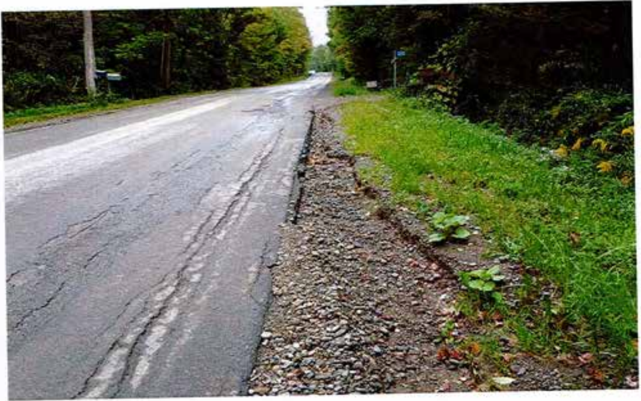
Osmun Road East lane and shoulder deterioration near 10200
