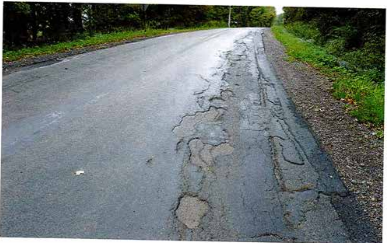
Osmun Road lane deterioration South of 10200
