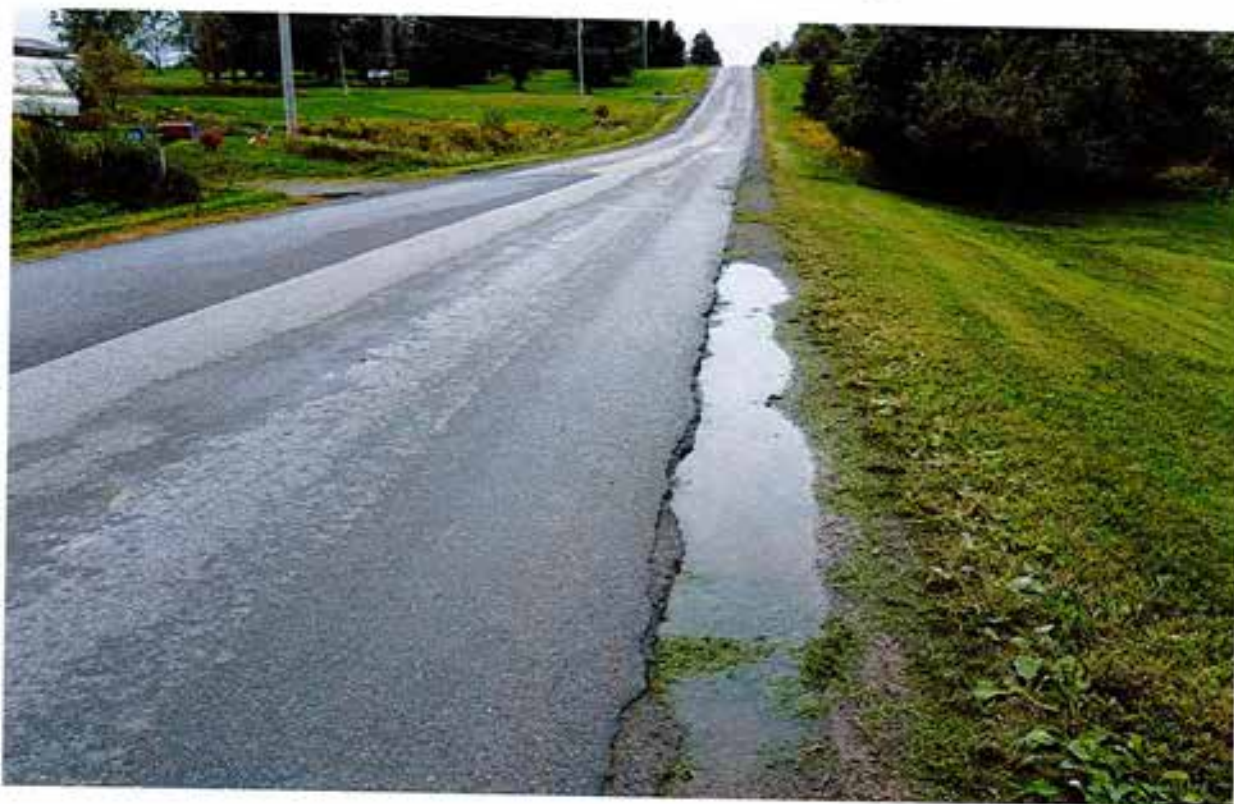
Bray Road North edge and shoulder deteriorating near 245
