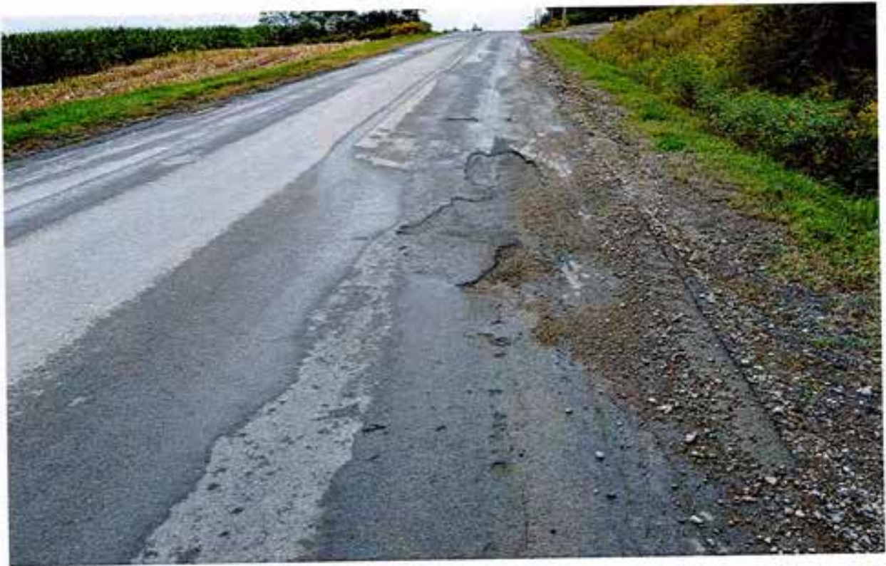
Bray Road lane deterioration near 2801 (#2)
