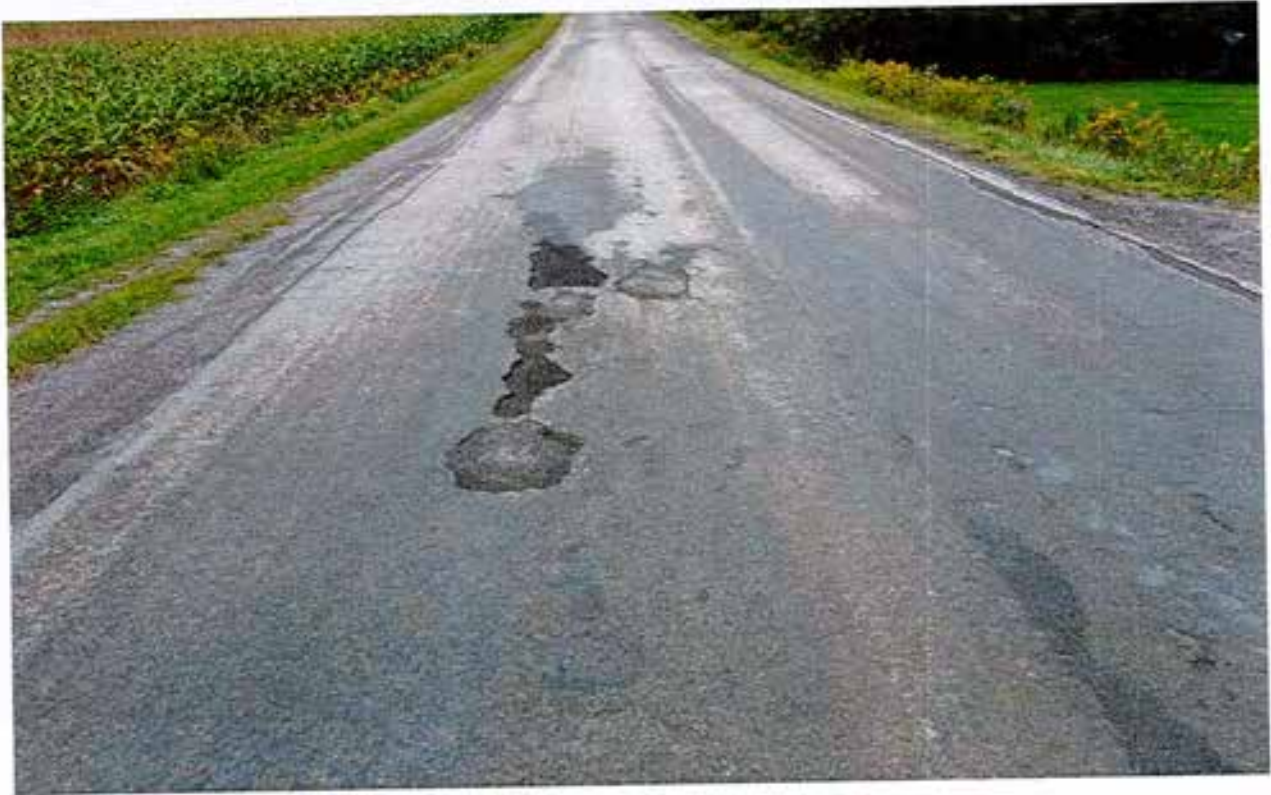
Osmun Road lane deterioration near 10674
