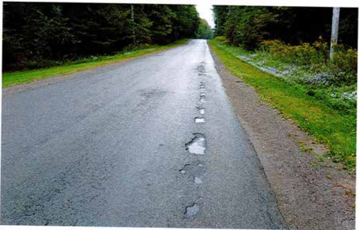
Eagle Street lane deterioration near 1000
