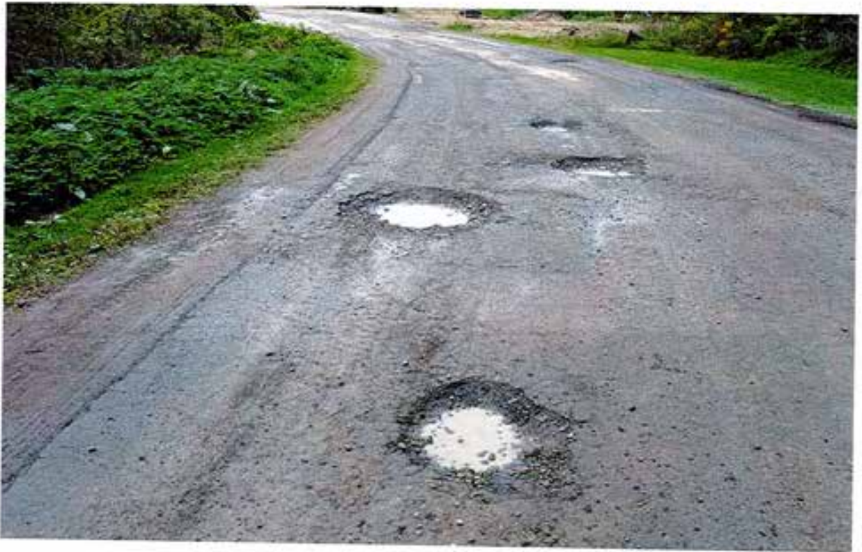
Strong Rd potholes
