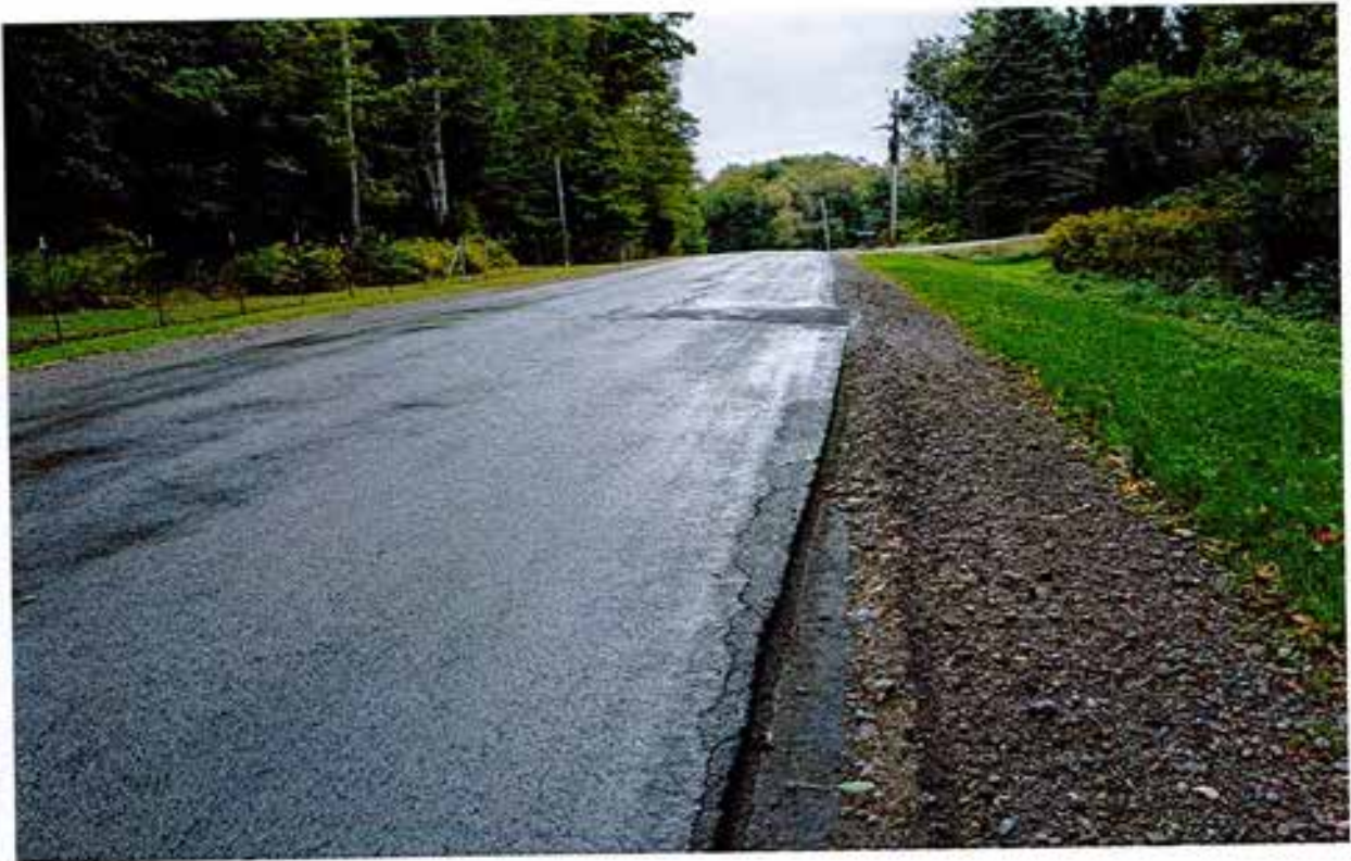
Eagle Street lane and shoulder deterioration near 1111
