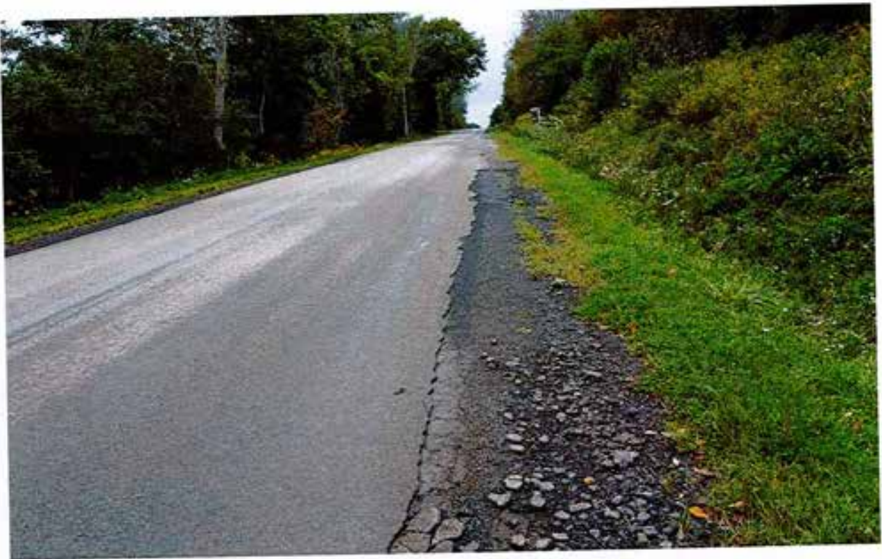
Osmun Rd East side lane, edge, and shoulder deterioration North and South of 10410
