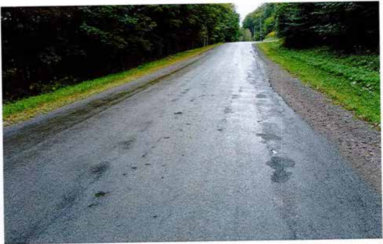
Eagle Street lane and edge deterioration near 931
