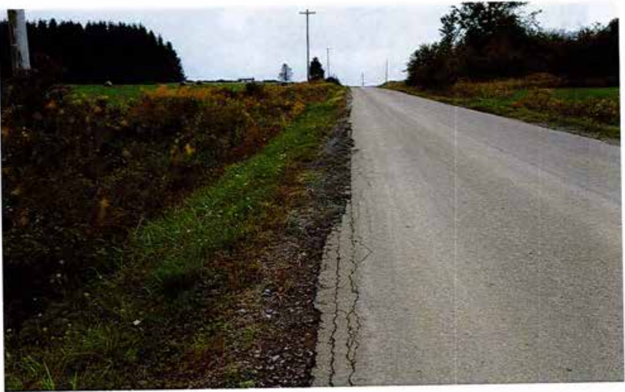
Galen Hill West edge and shoulder deterioration North of 10075
