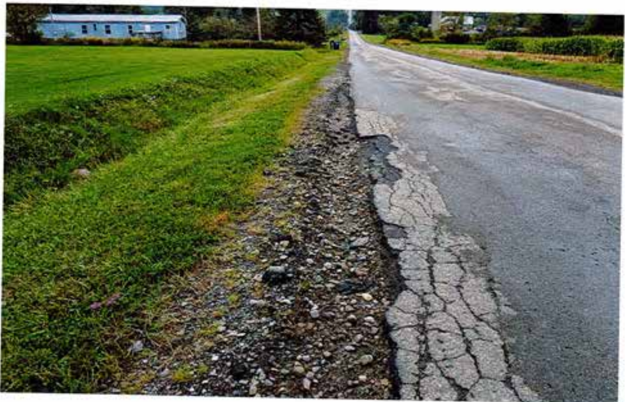
Bray Road South edge and shoulder deteriorating near 409
