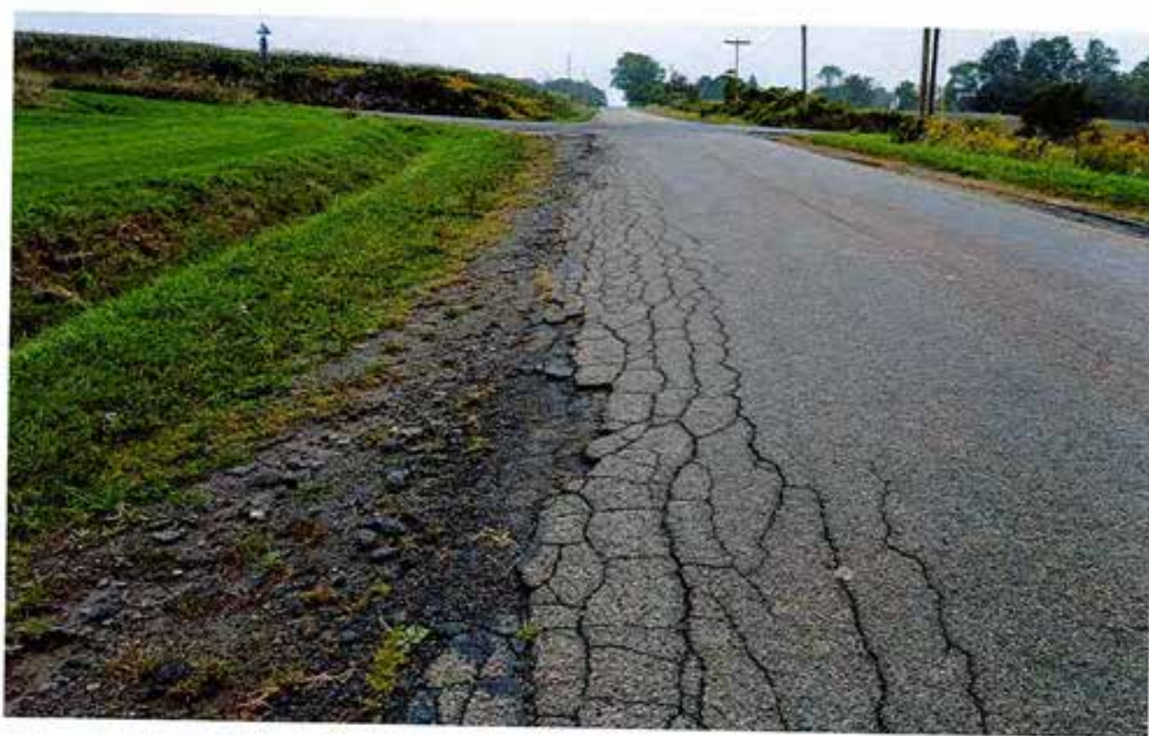
Sandbank Road (East and West) edge and shoulder deteriorating near intersection with Cross Road
