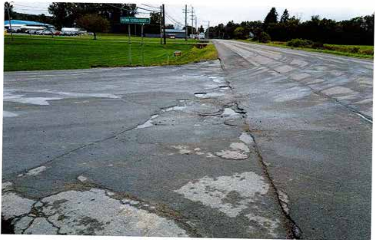
Brown Schoolhouse Road lane deterioration near intersection with Route 98
