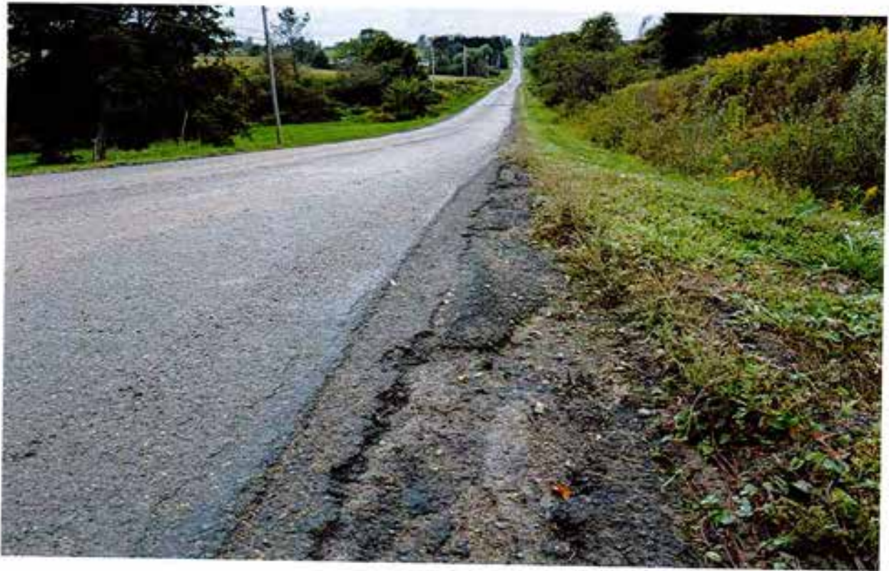
Bray Road North edge and shoulder deteriorating from +/-113 to +/-2473
