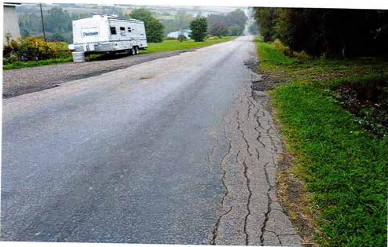
Sandbank Rd East and West side shoulder deterioration near 10442
