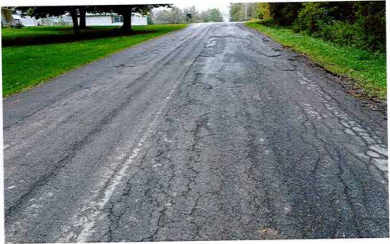
Sandbank Rd lane deterioration near 10317
