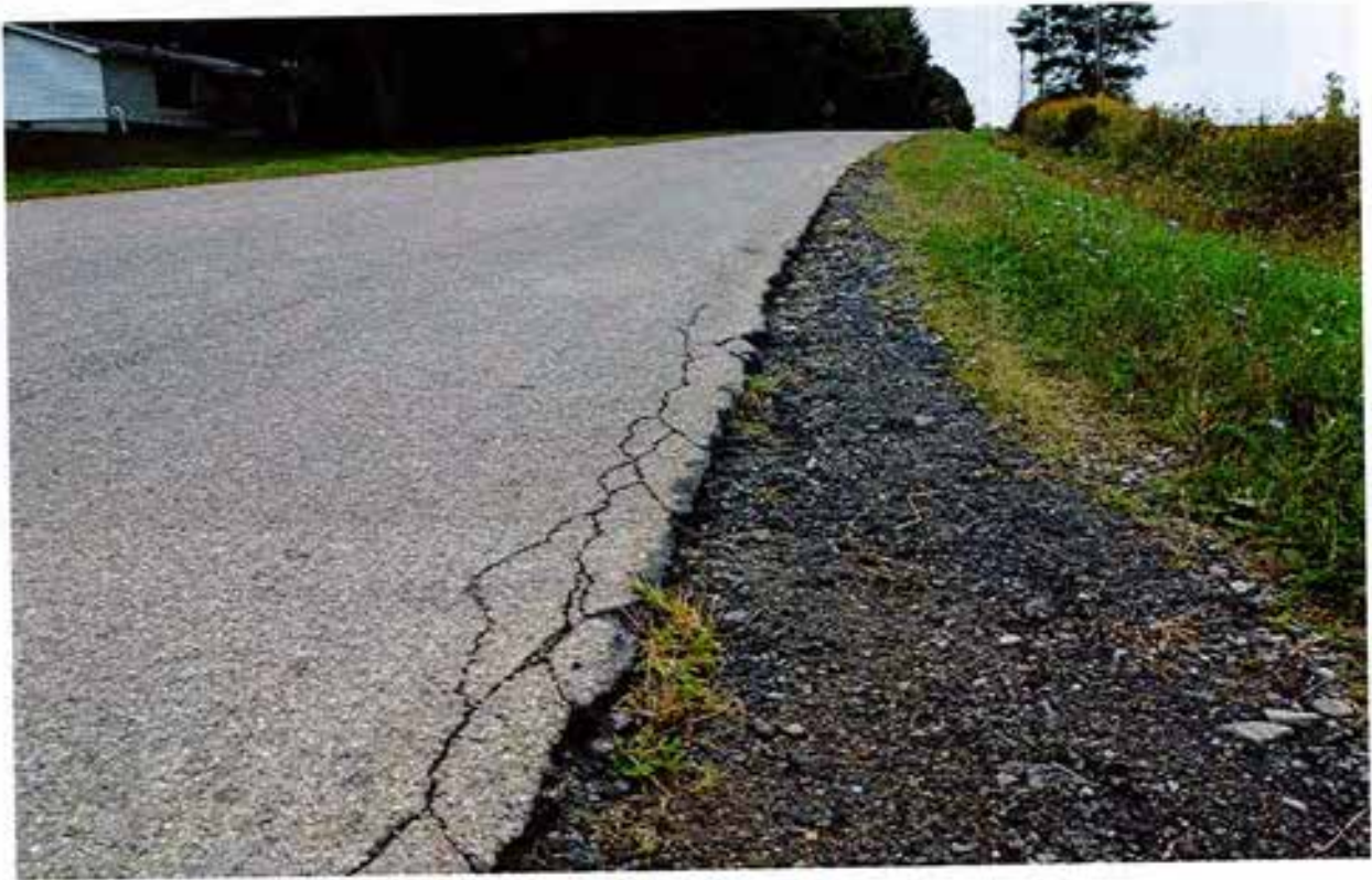
Edmunds Rd Southeast edge and shoulder deteriorating near 1812
