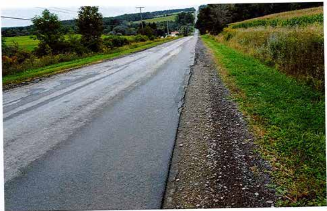
Bray Road North edge and shoulder deteriorating from 475 to Eagle Street
