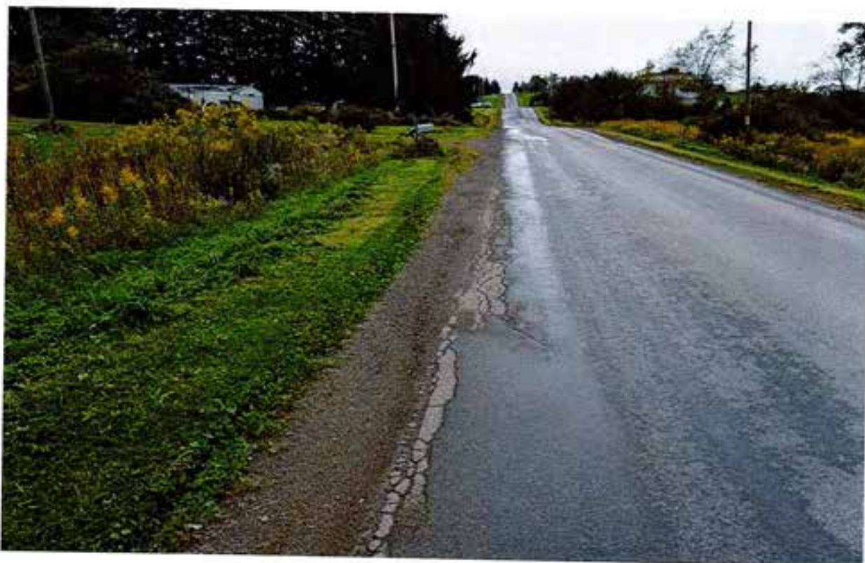
Bray Road South edge and shoulder deteriorating near 223
