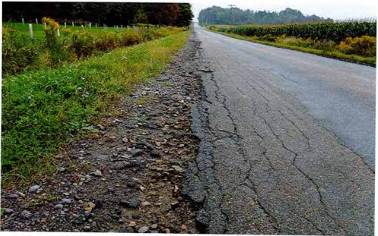
Baird Road North edge deterioration from +/- 379 to +/- 253
