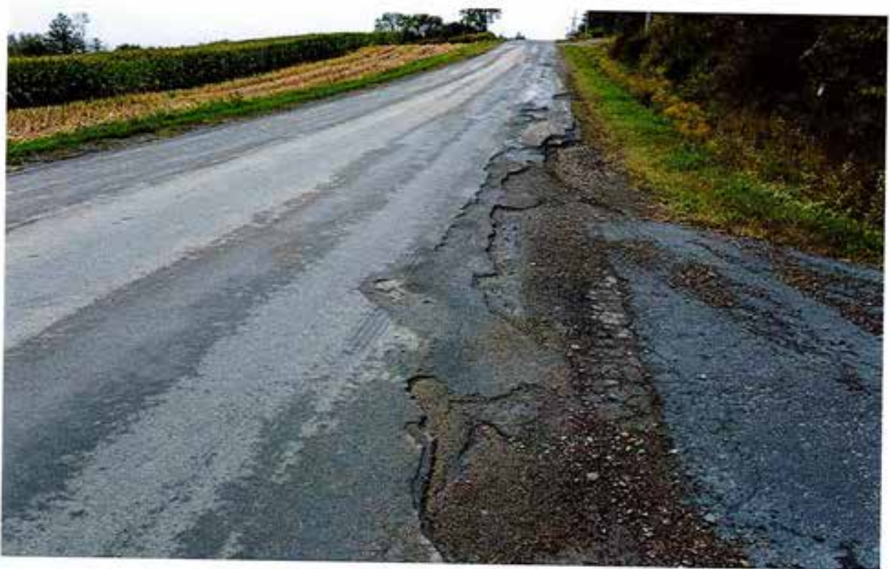
Bray Road North edge and lane deterioration near 2801 (#1)
