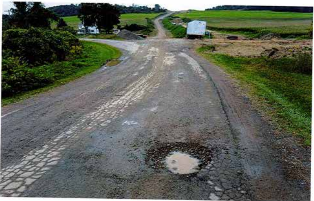
Strong Road pothole
