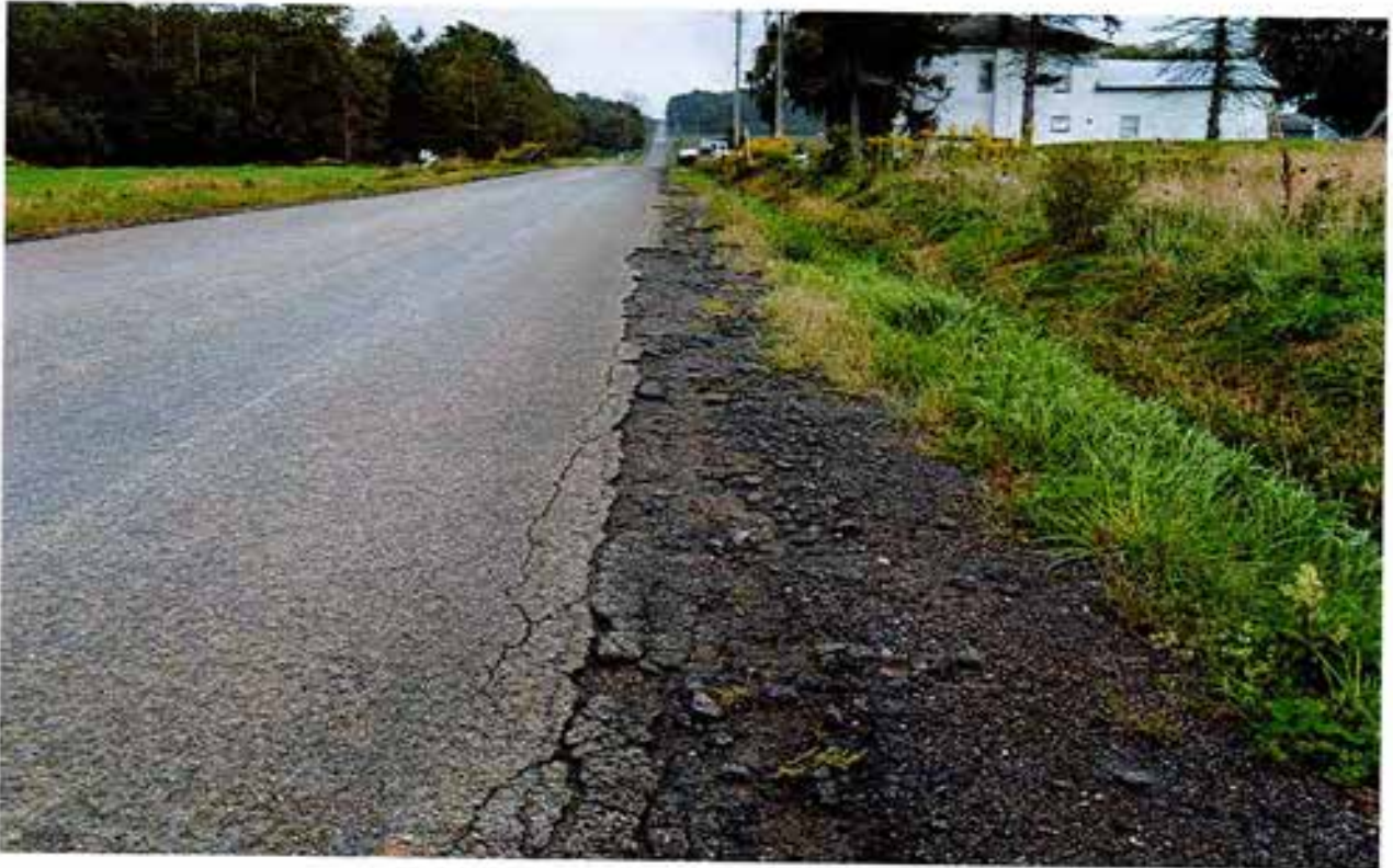
Baird Rd South shoulder deterioration East and West of 379
