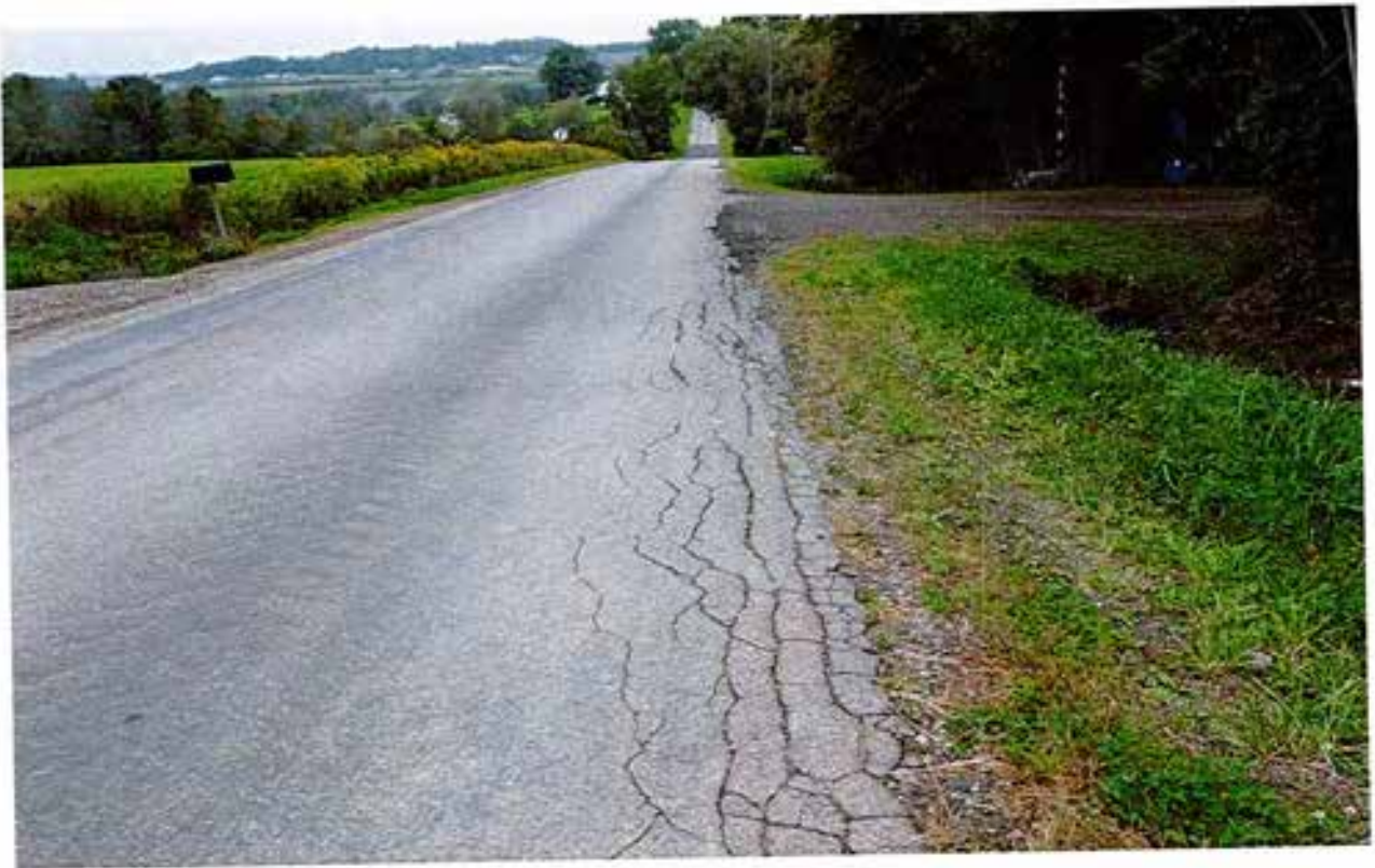
Sandbank Road East and West edge / shoulder deterioration near 10238
