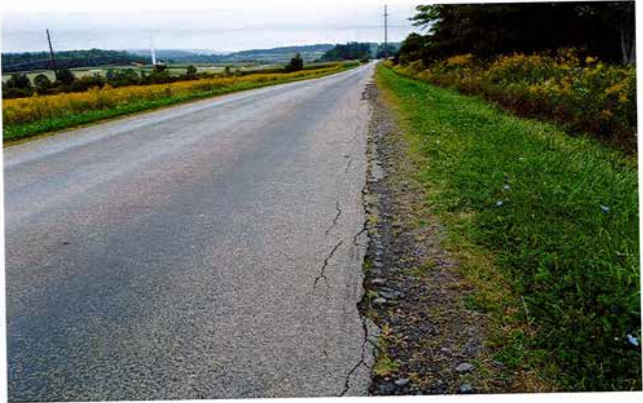
Sandbank Rd East and West edge deterioration North and South of 10157 to +/- 10220
