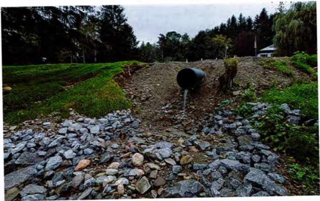
Osmun Rd: West end of Culvert near 10379. Consider rock revetment (rock lining) alongside slope from the road to prevent further washout of this slope.
