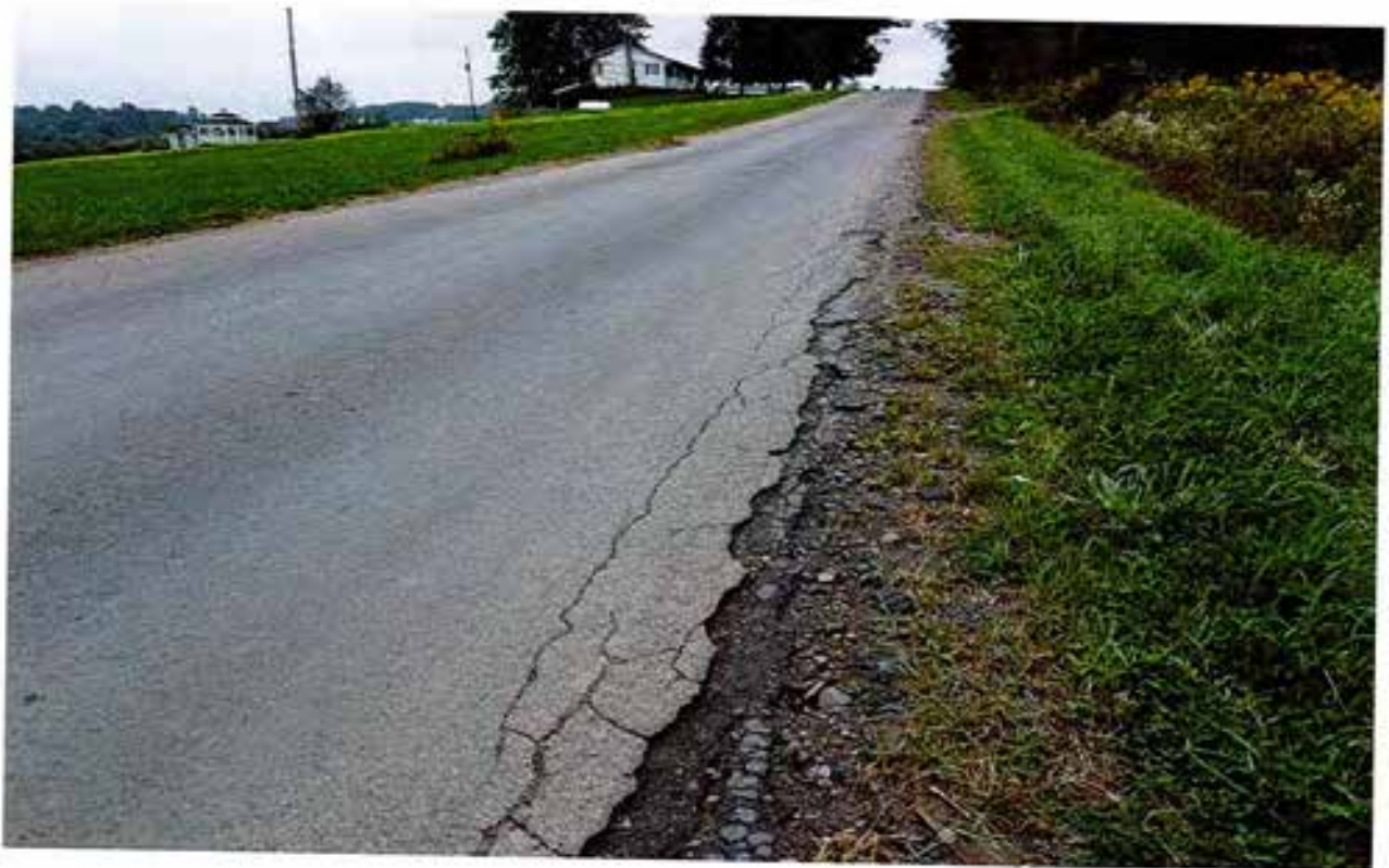
Sandbank Rd East lane and edge deterioration South of 10317
