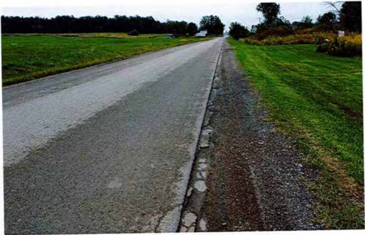
Brown Schoolhouse Road West shoulder deterioration from 11354 to 11258
