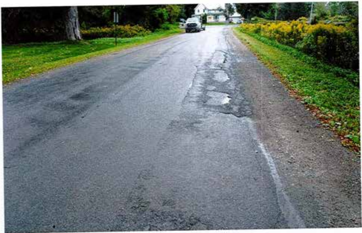
Eagle Street East lane deterioration near 708
