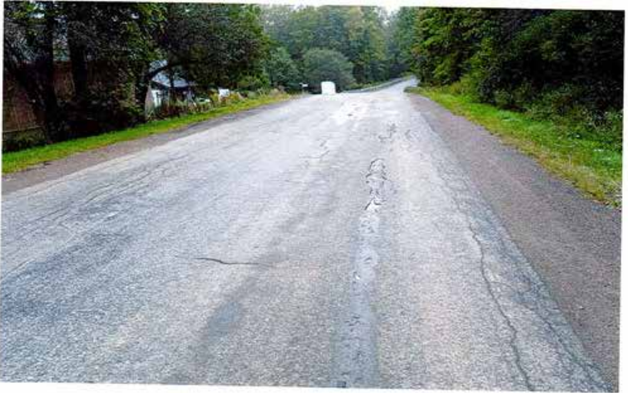
Osmun Rd lane deterioration near Zimmer
