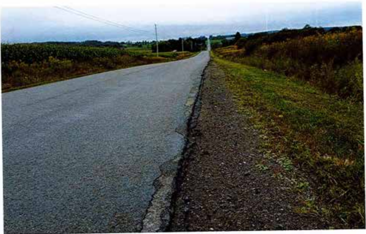
Bray Road North edge and shoulder deteriorating from gas pipeline #57 to +/- House 113
