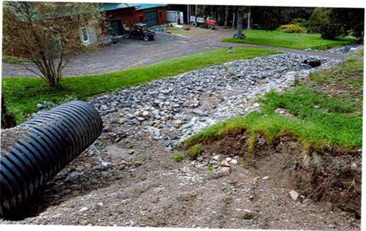
Osmun Rd: West side of Culvert near 10379. Exposed side slope subject to washout.
