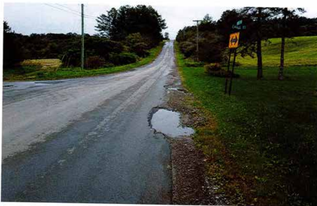
Bray Road Edge Deterioration at Eagle Street Intersection
