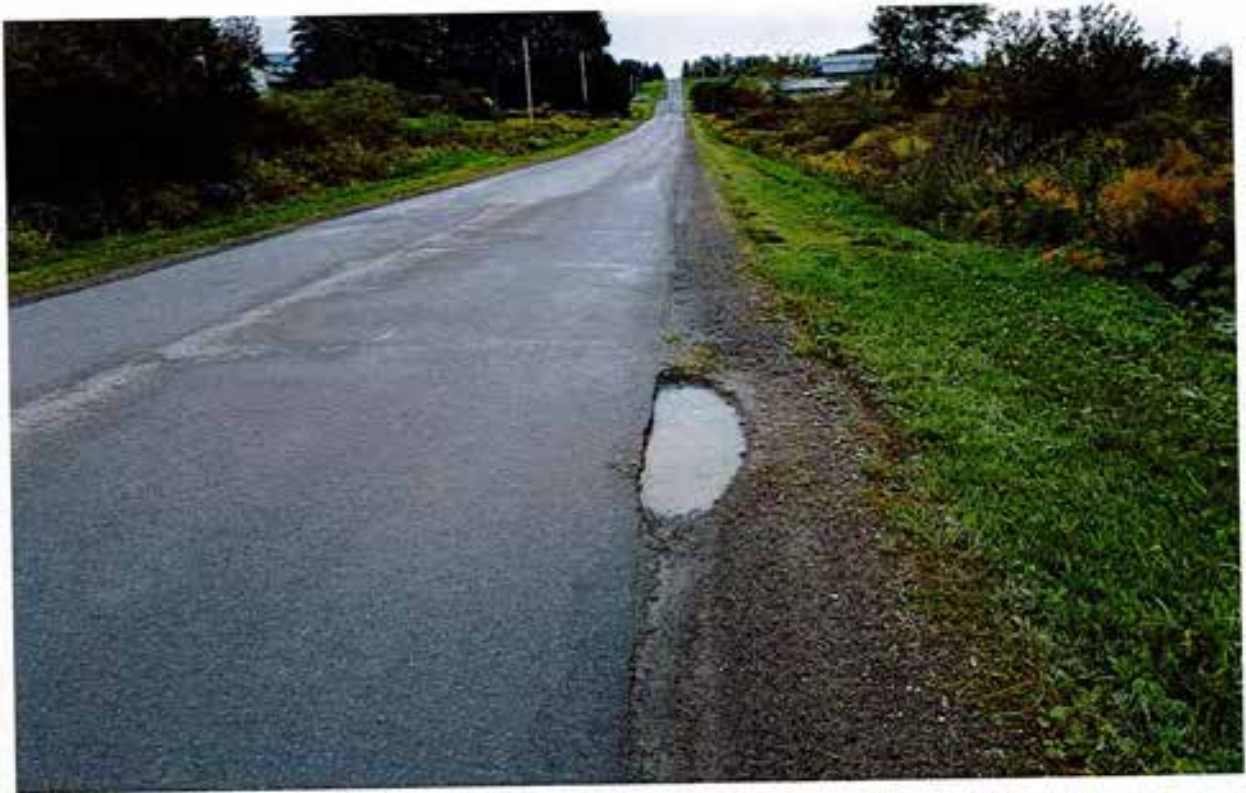
Bray Road North edge and shoulder deteriorating with Pothole near 2407
