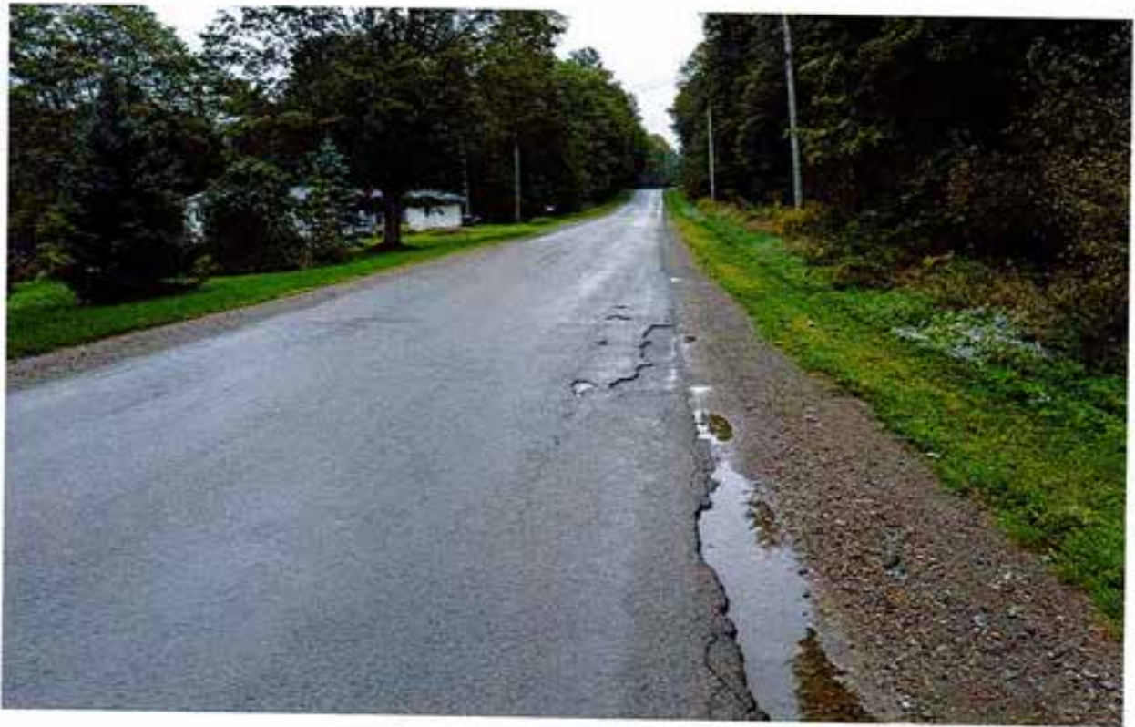
Eagle Street lane and East edge deterioration near 994
