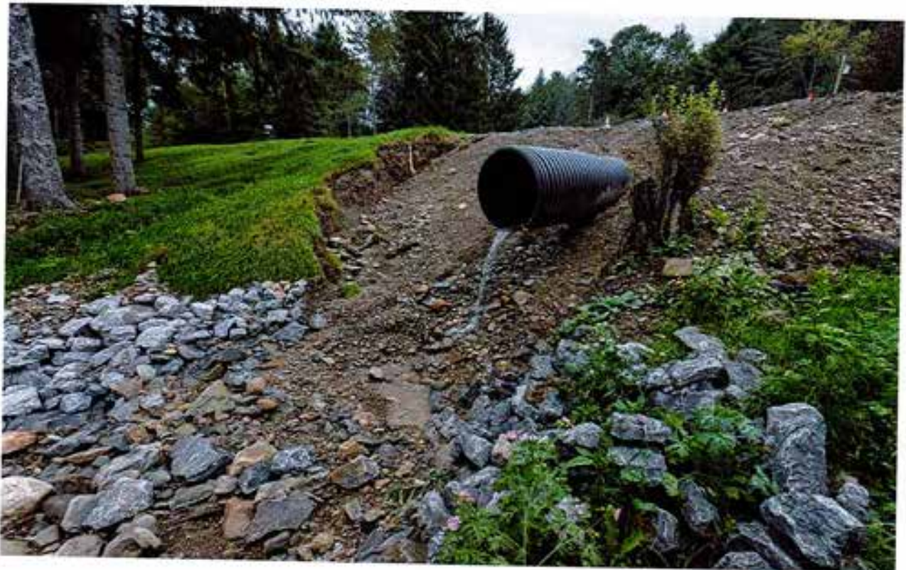
Osmun Rd: West end of Culvert near 10379. Recommend cutting pipe back to daylight grade and installing rock outlet protection to prevent further erosion of outlet area.
