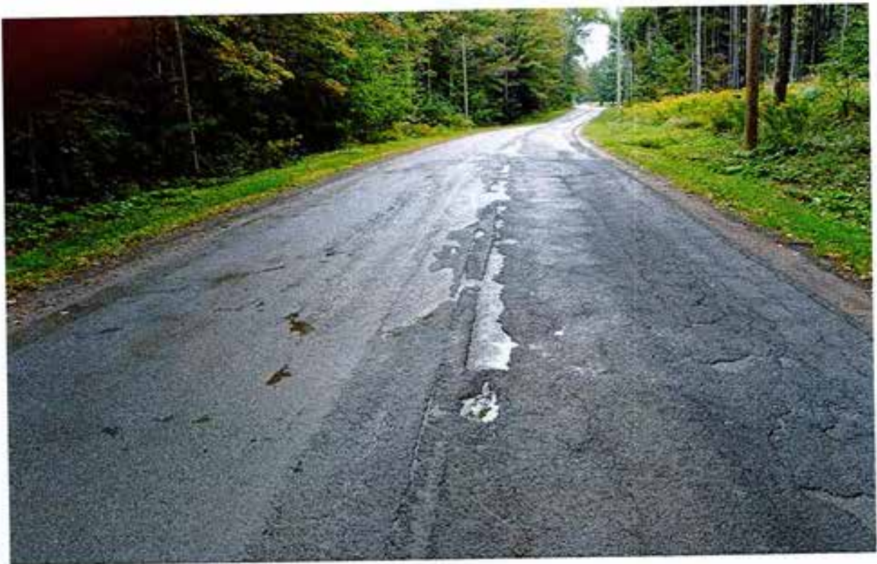
Eagle Street lane deterioration near 915
