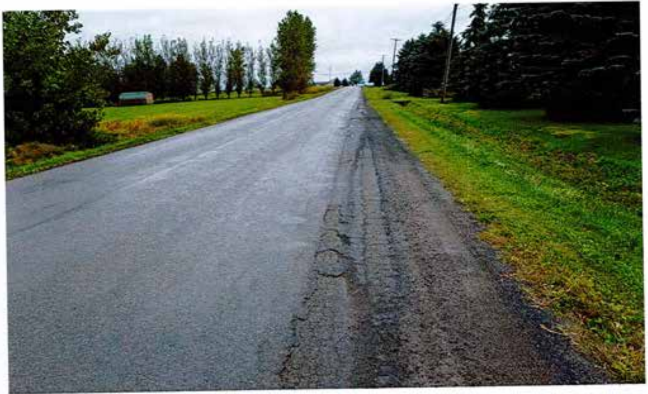
North Road lane, edge, and shoulder deterioration near 11980
