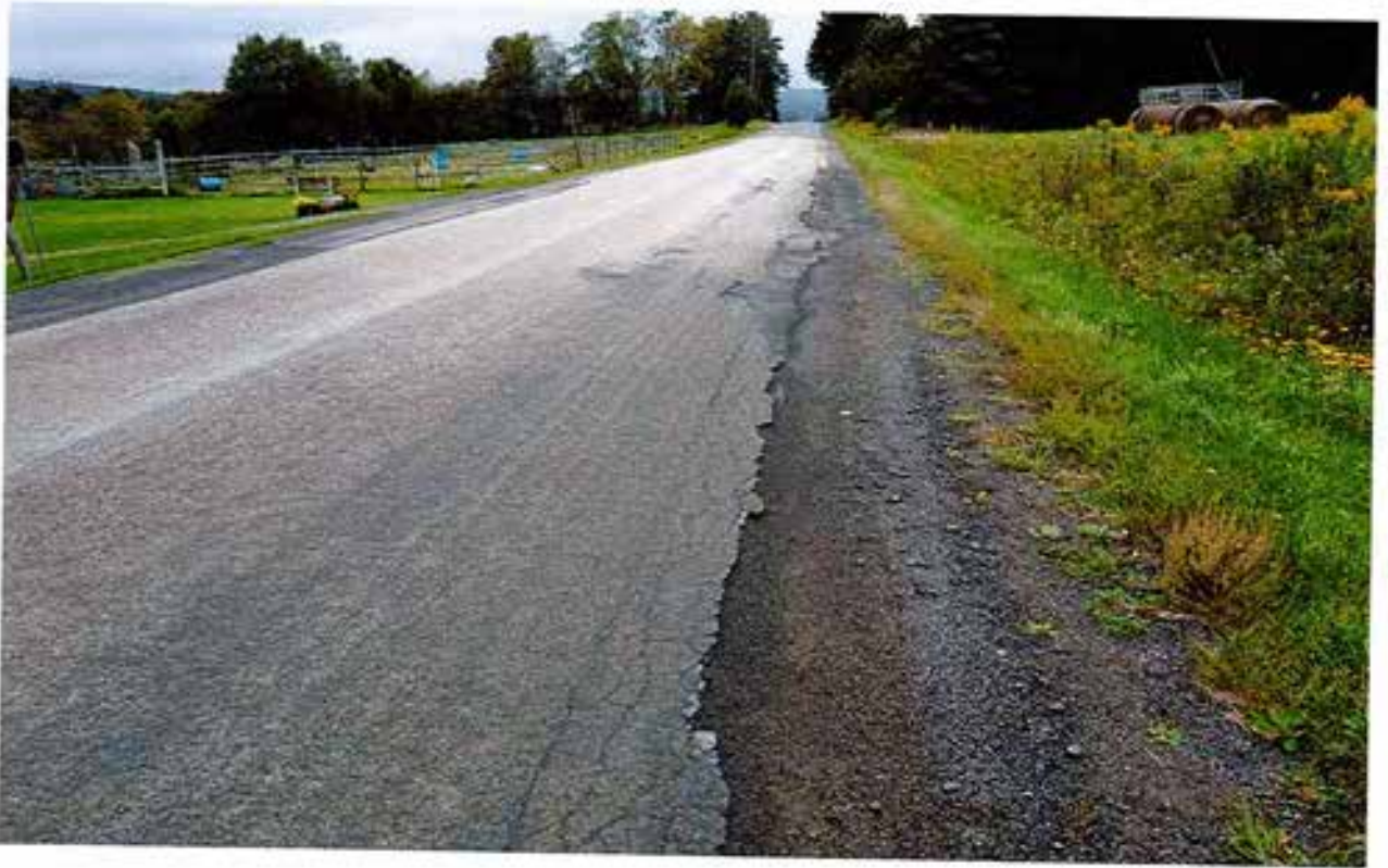
Osmun Road East edge and shoulder deterioration near 10571
