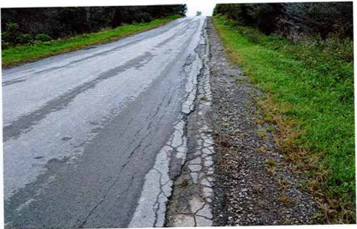
Bray Road North edge and shoulder deteriorating from Eagle Street to +/- 2801
