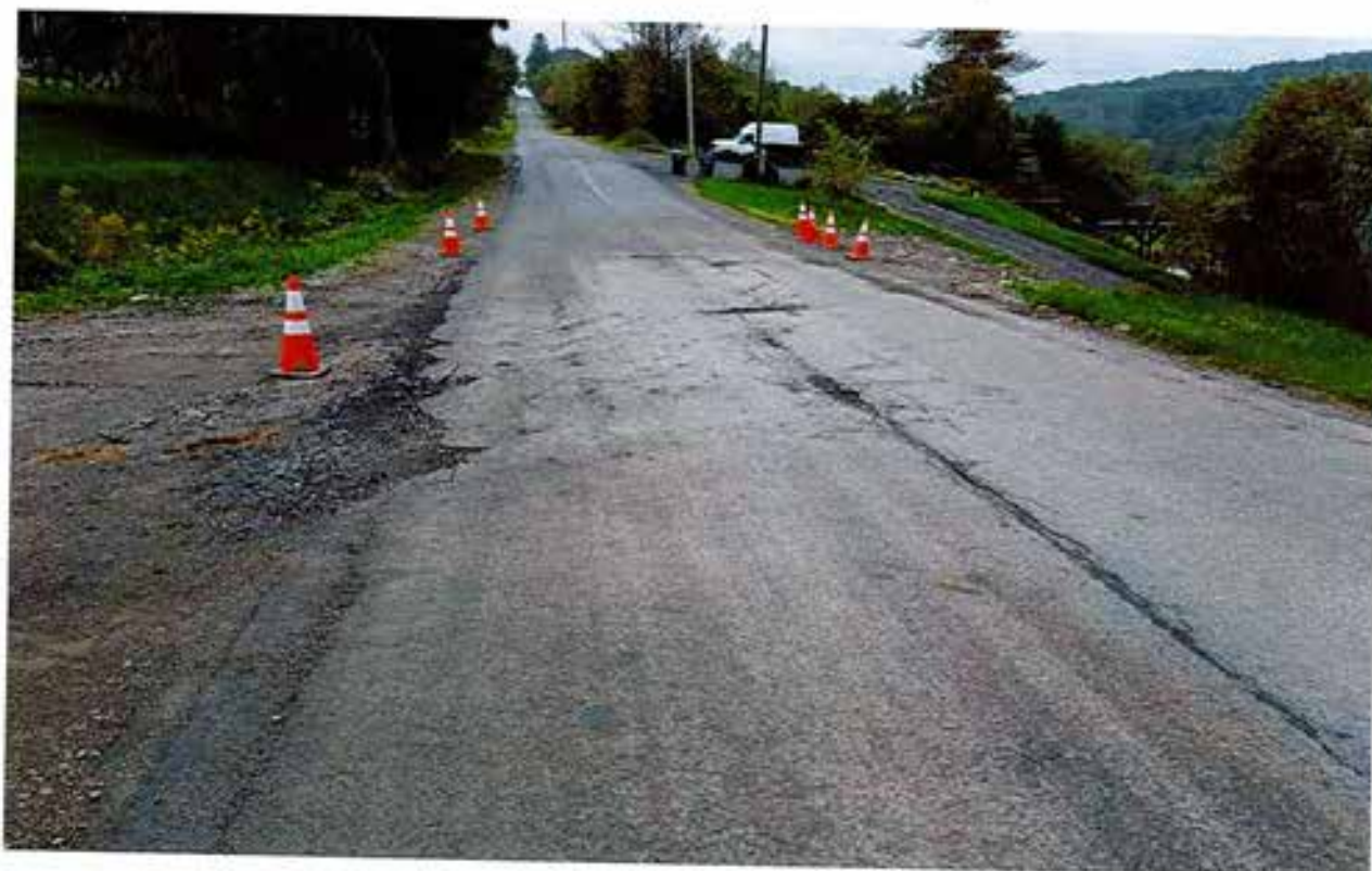
Osmun Rd: Road over Culvert near 10379 facing South. Road edge deterioration is evident.
