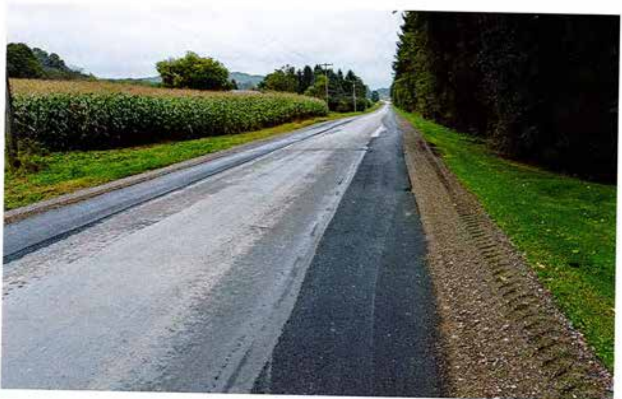
Siloam Road North and South shoulder deterioration from +/- 1675 to +/- 1579 (REPAIRED)
