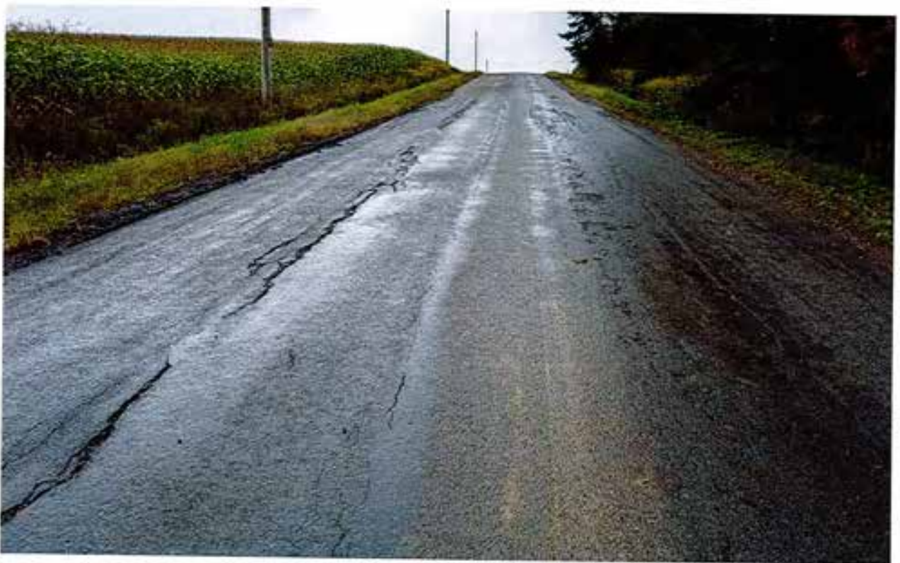
Baird Road lane deterioration from 253 to 187
