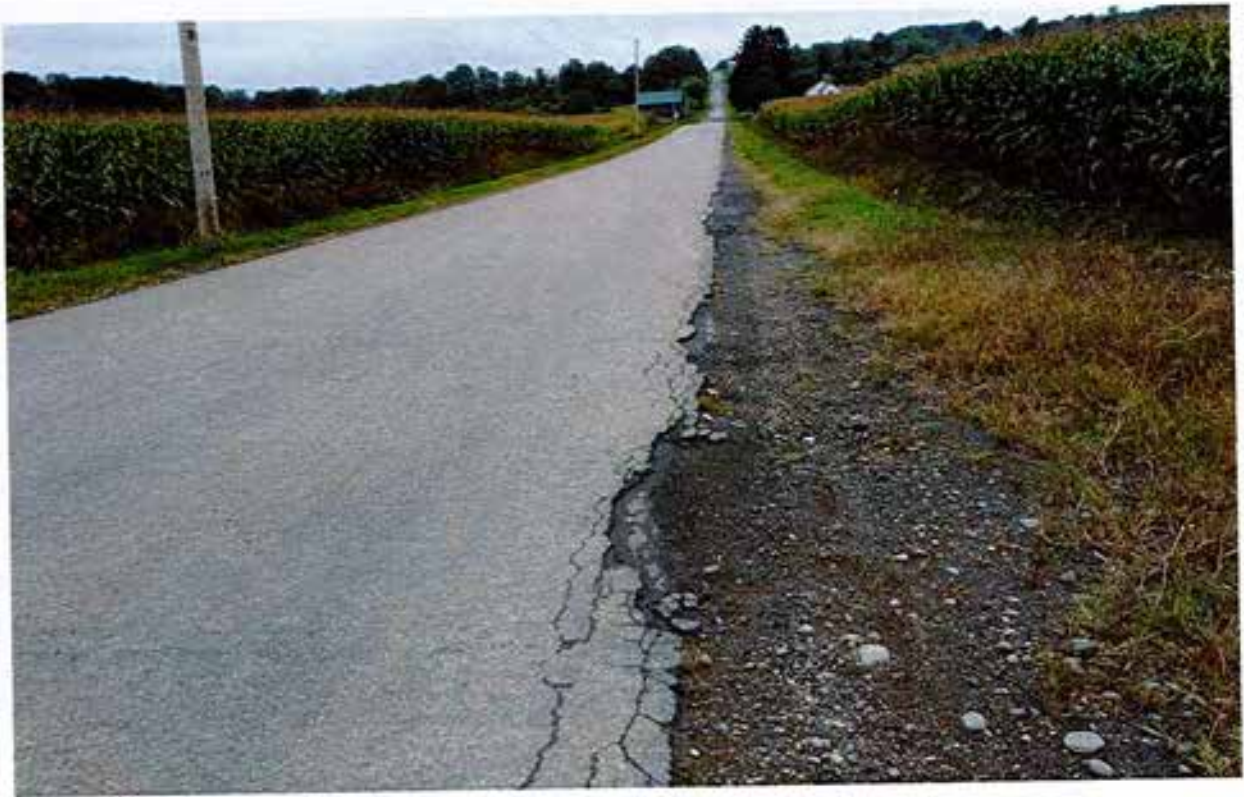
Fisher Blake Road North edge and shoulder deterioration from 2195 to +/- 2272
