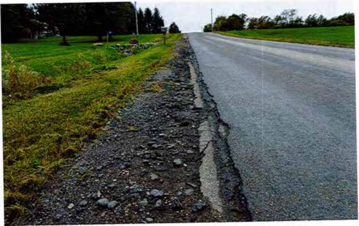
Bray Road South edge and shoulder deteriorating near 259
