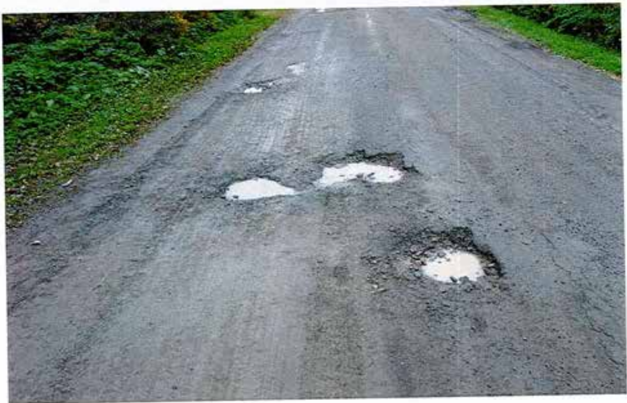
Strong Road potholes
