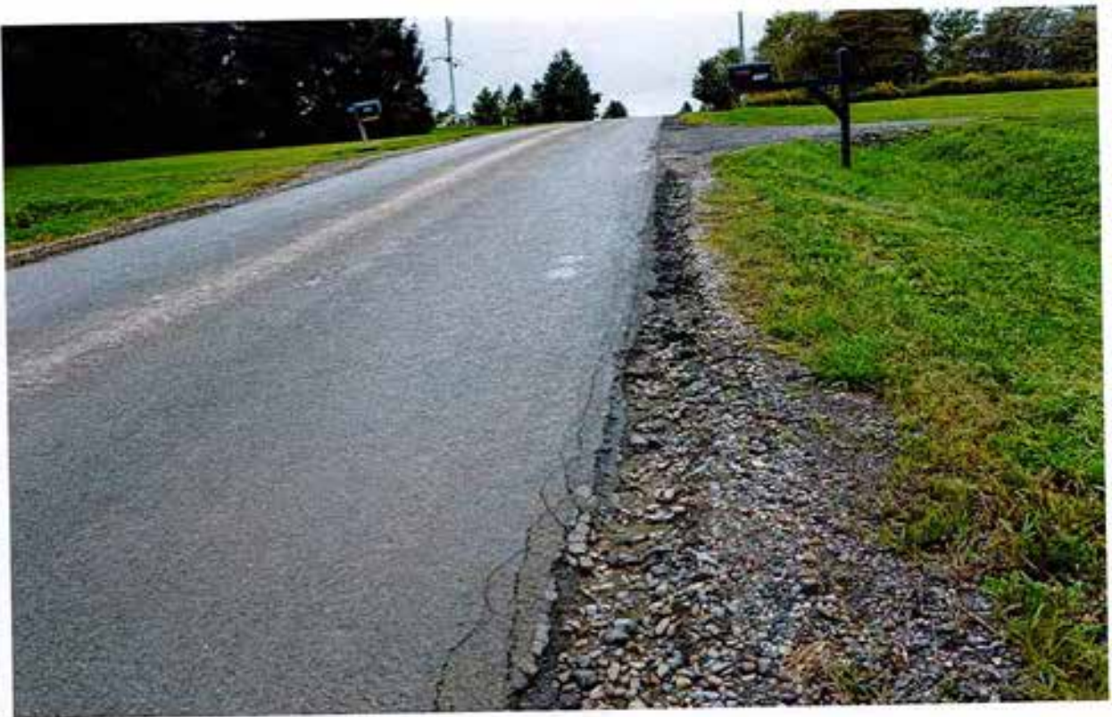
Bray Road North edge and shoulder deteriorating near 2317
