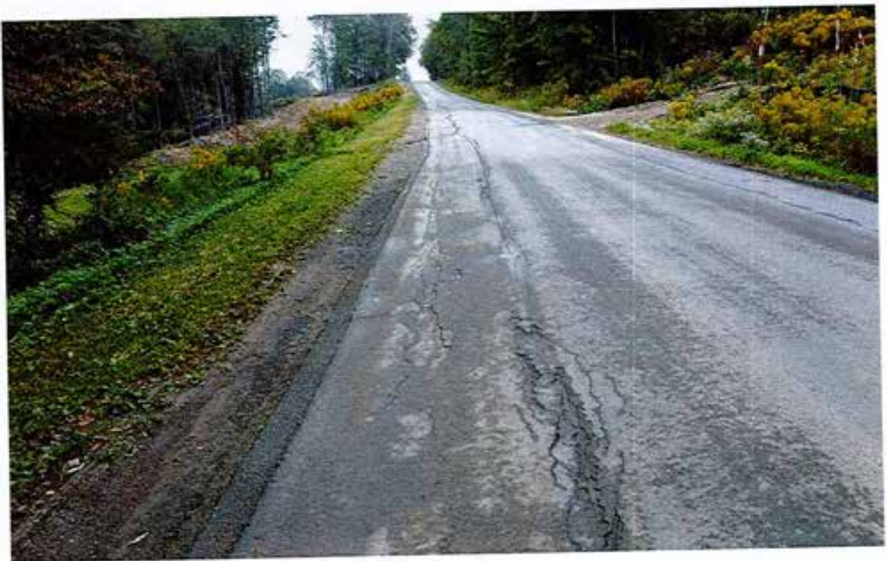
Osmun Rd lane deterioration North of 10220 near construction entrance
