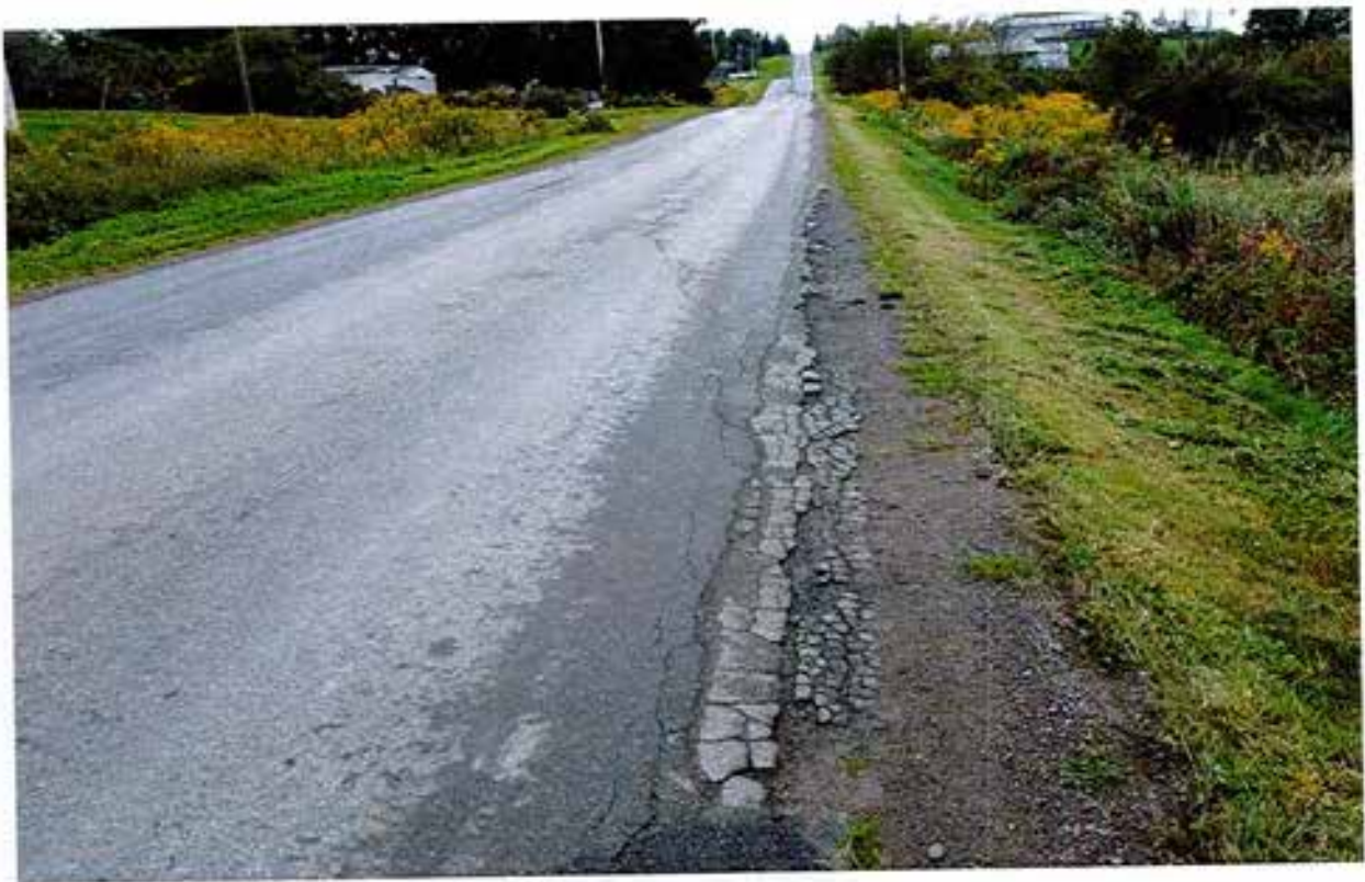
Bray Road North edge deteriorating near 223
