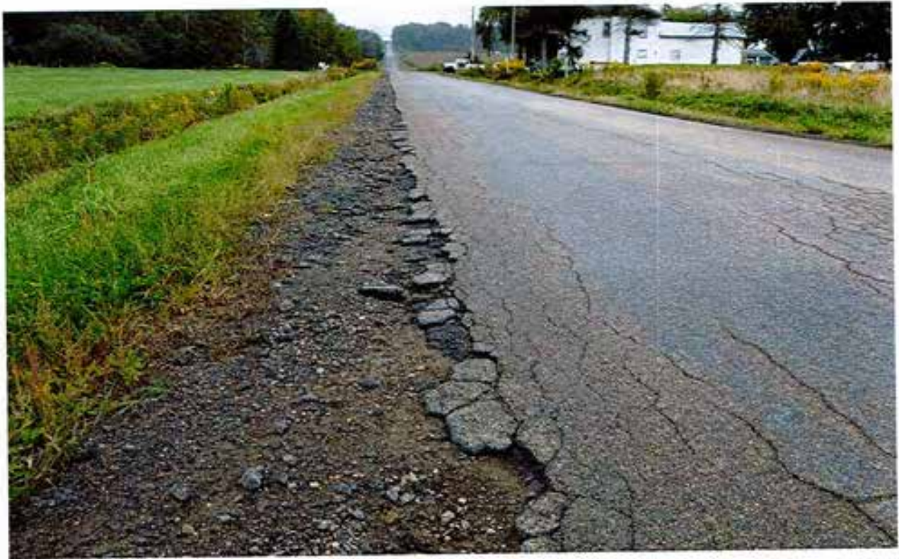
Baird Rd North shoulder deterioration East and West of 379
