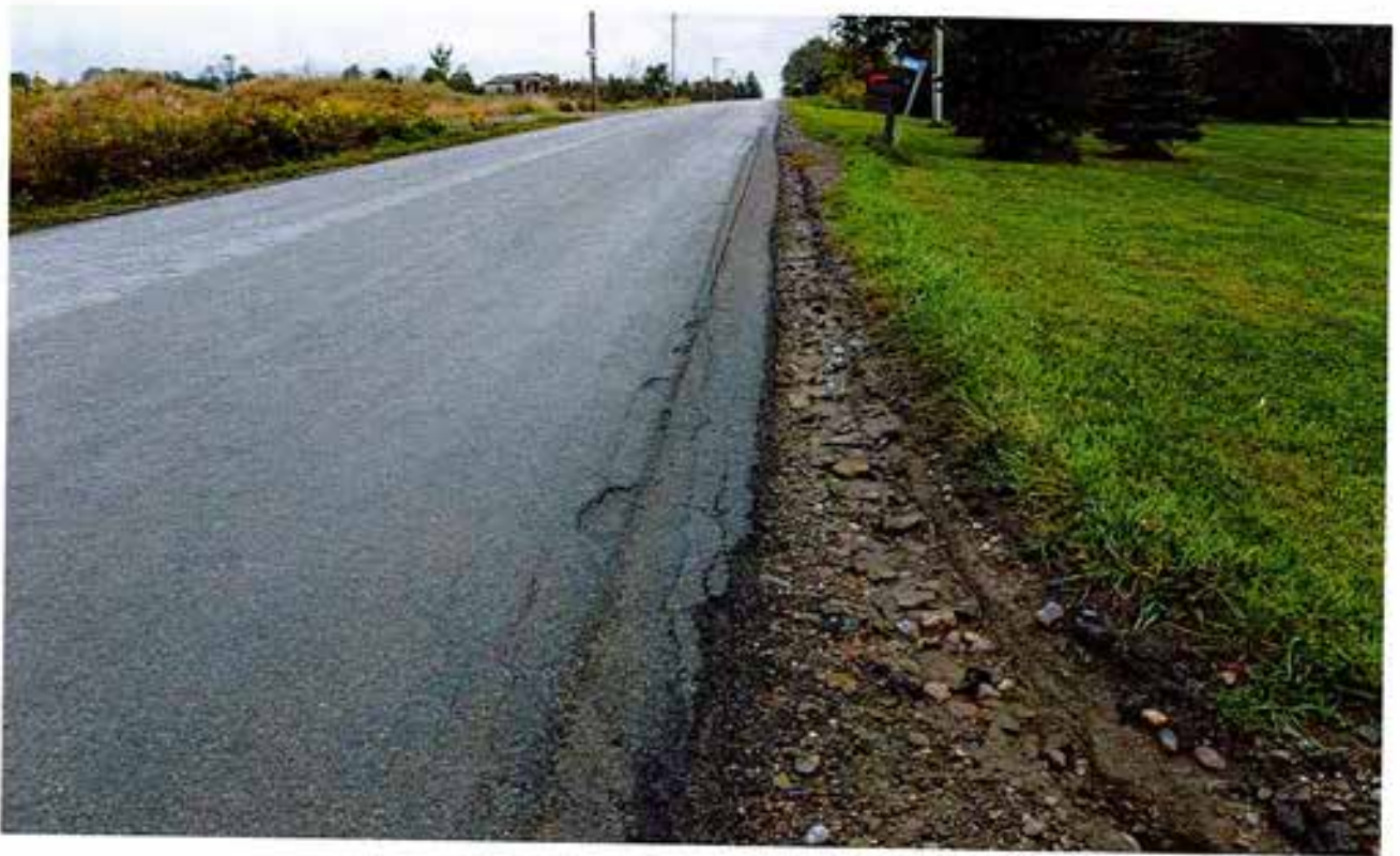
North Road North edge and shoulder deterioration near 11614
