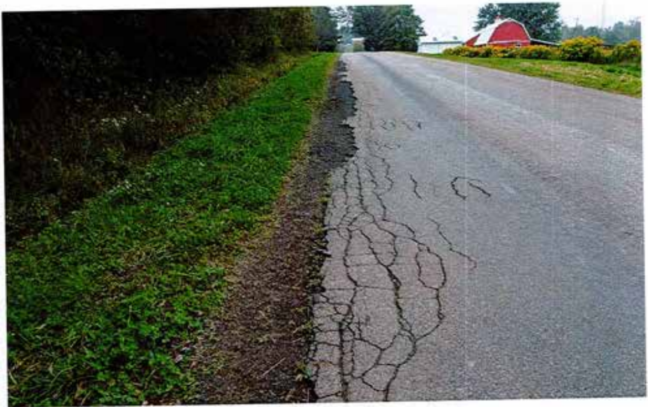
Sandbank Road East edge deterioration South of 10368
