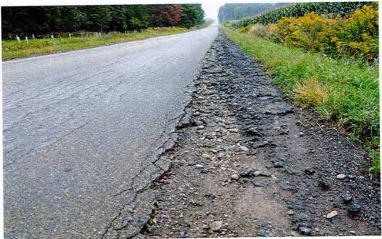
Baird Road South edge deterioration from +/- 379 to +/- 253
