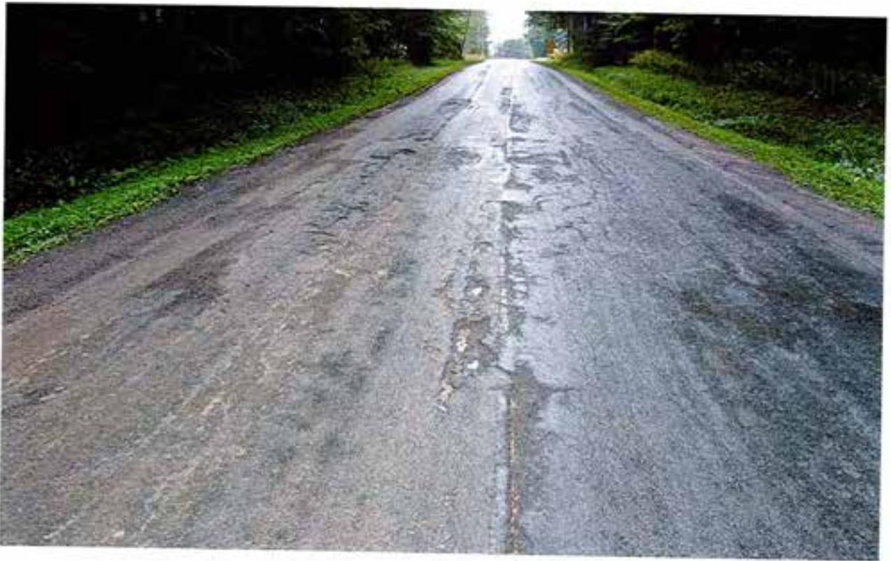
Galen Hill Road lane deterioration from Phillippi Rd to 10553
