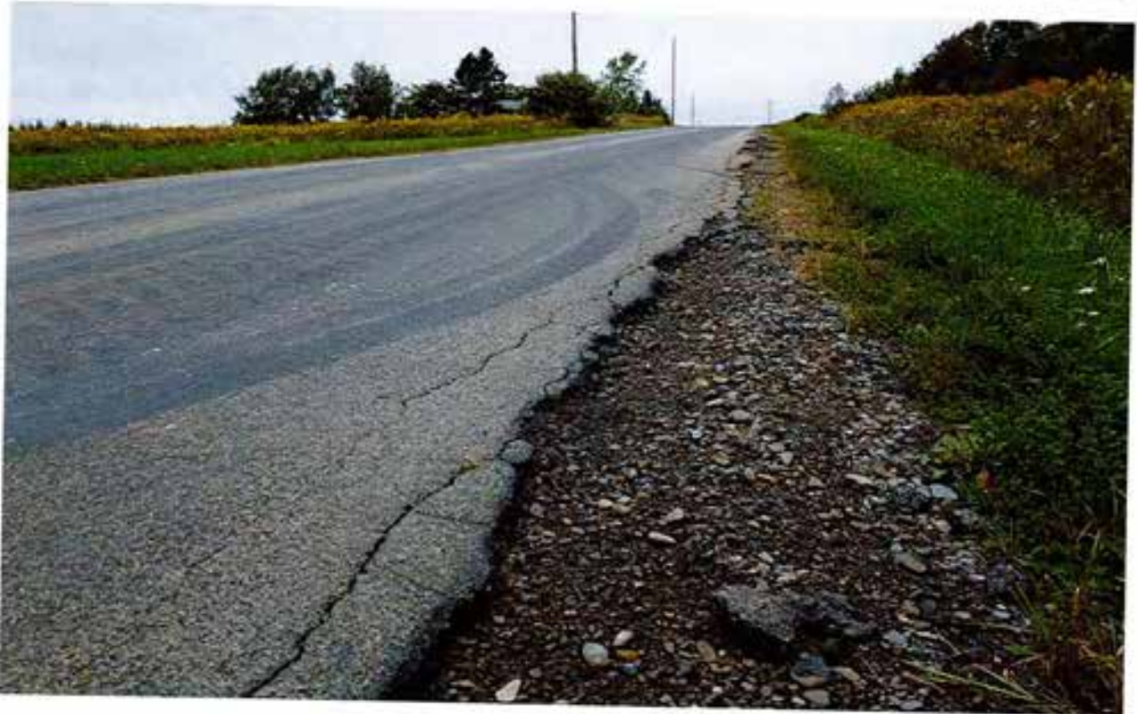
Sandbank Road East edge and shoulder deterioration near 9999
