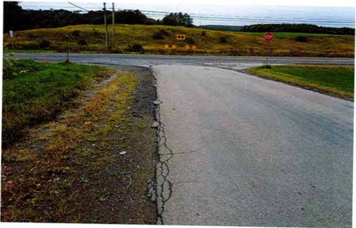
Edmunds Rd lane and shoulder deterioration on North and South sides of Rd near intersection with Maple Grove
