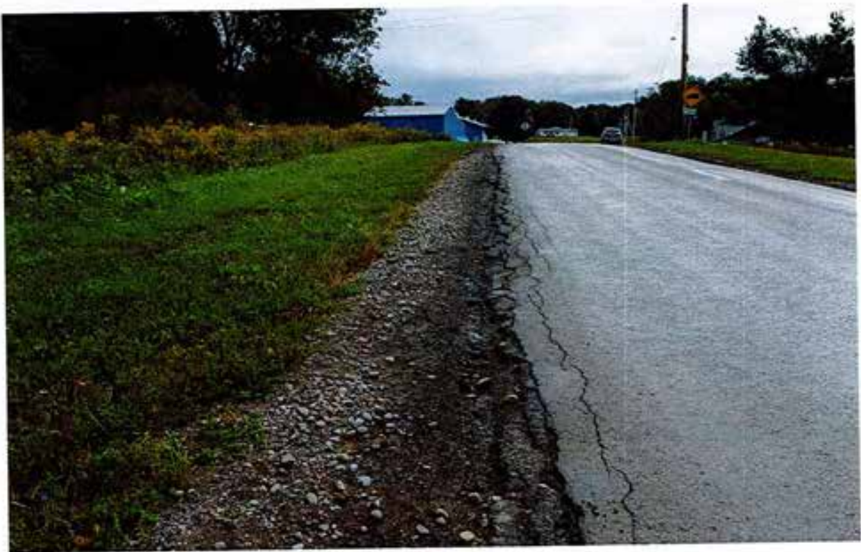
Eagle Street North and South side lane and edge deterioration near 1219
