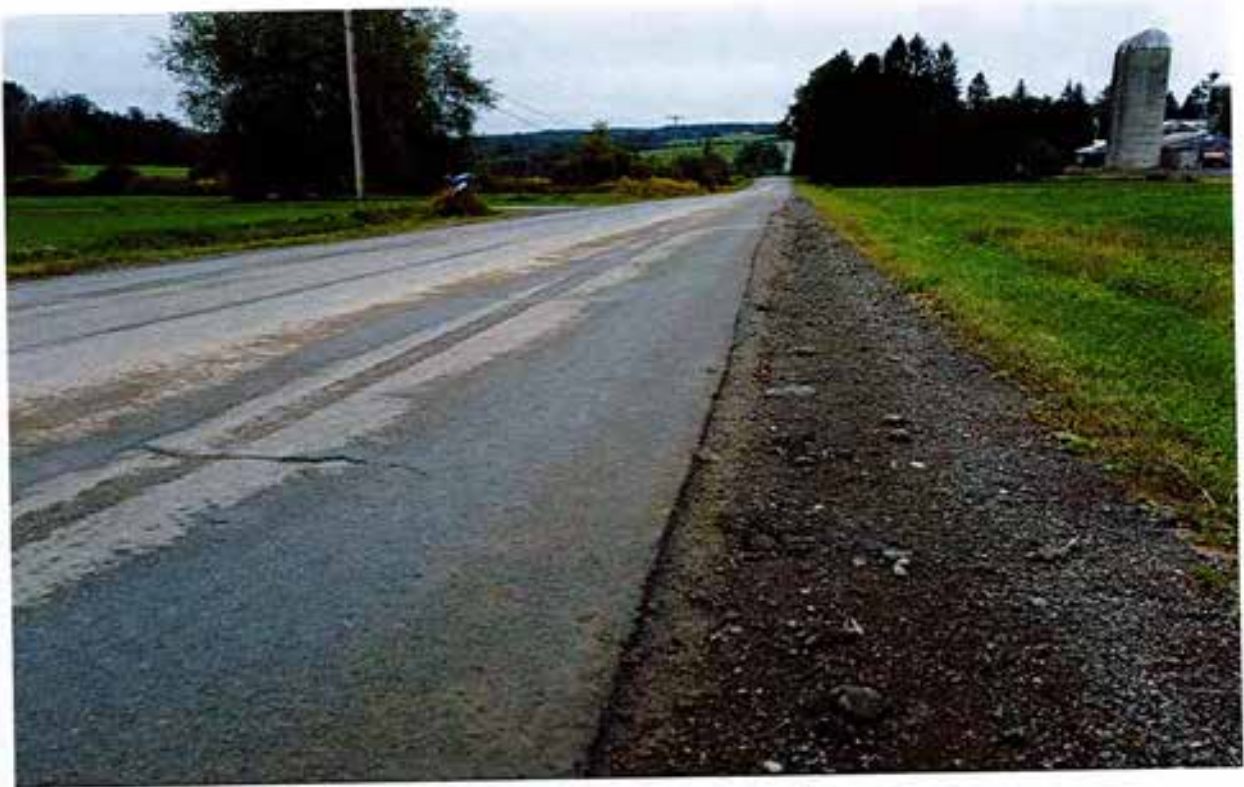
Bray Road North edge and shoulder deteriorating from 445 to 475
