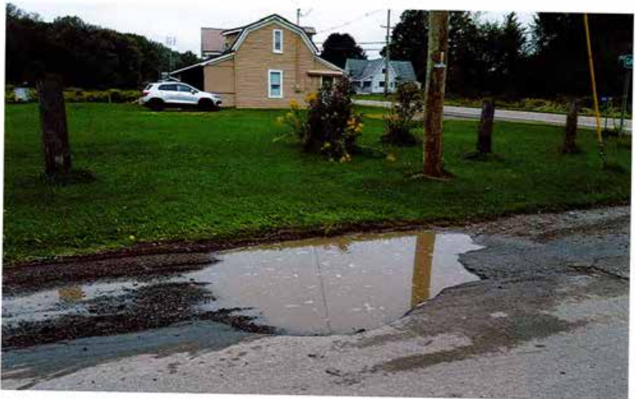
Galen Hill Rd pothole at intersection of Route 98
