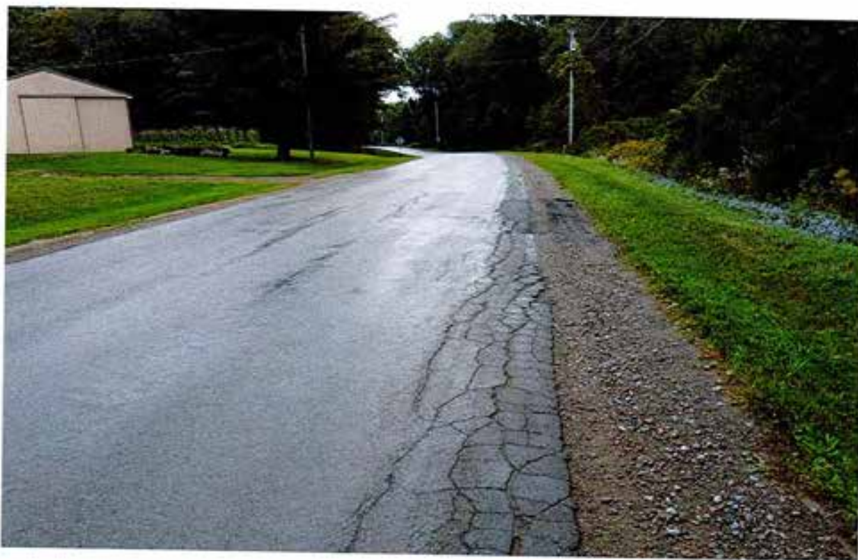
Eagle Street lane and edge deterioration near 1152
