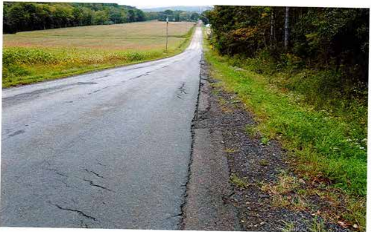
Osmun Rd edge deterioration South of 10674
