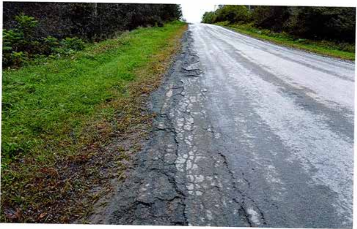
Bray Road South edge and shoulder deteriorating from Eagle Street to +/- 2801
