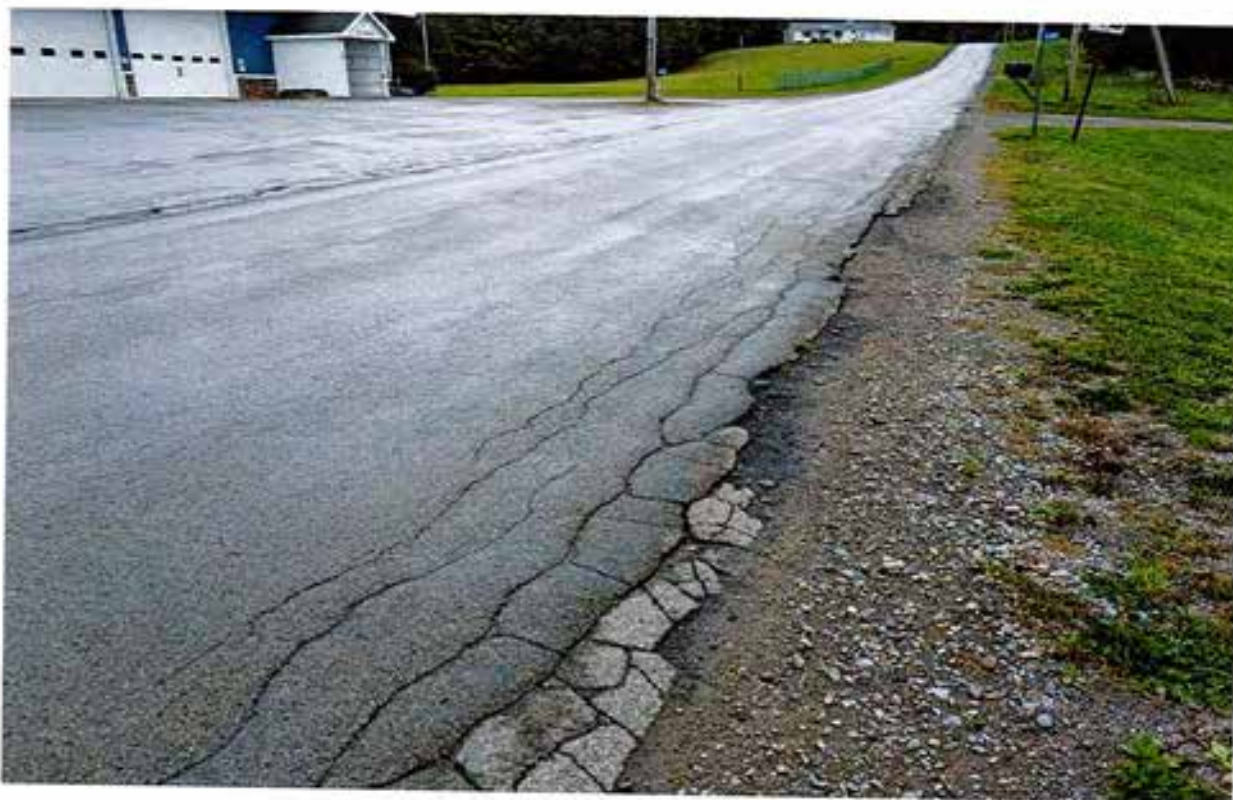
Eagle Street South side lane and edge deterioration near 11405
