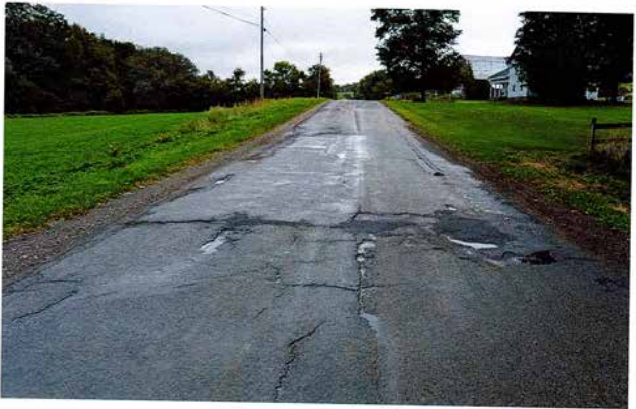
Eagle Street lane deterioration South of 849
