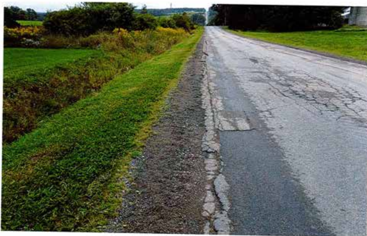
Bray Road South edge and shoulder deteriorating from 475 to Eagle Street
