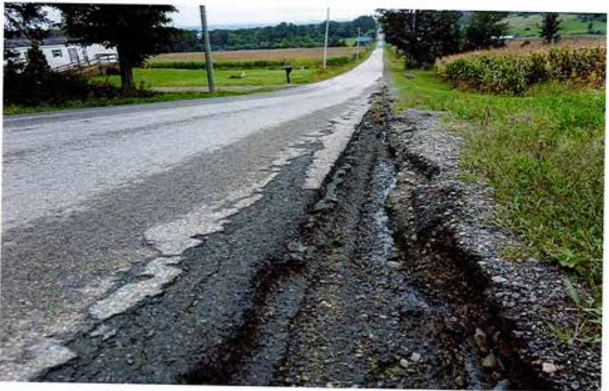
Fisher Blake Road North edge and shoulder deterioration near 2195
