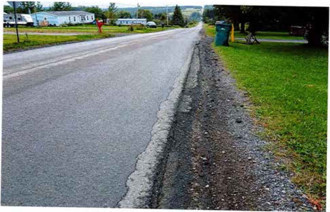
Bray Road North edge and shoulder deteriorating near 2231
