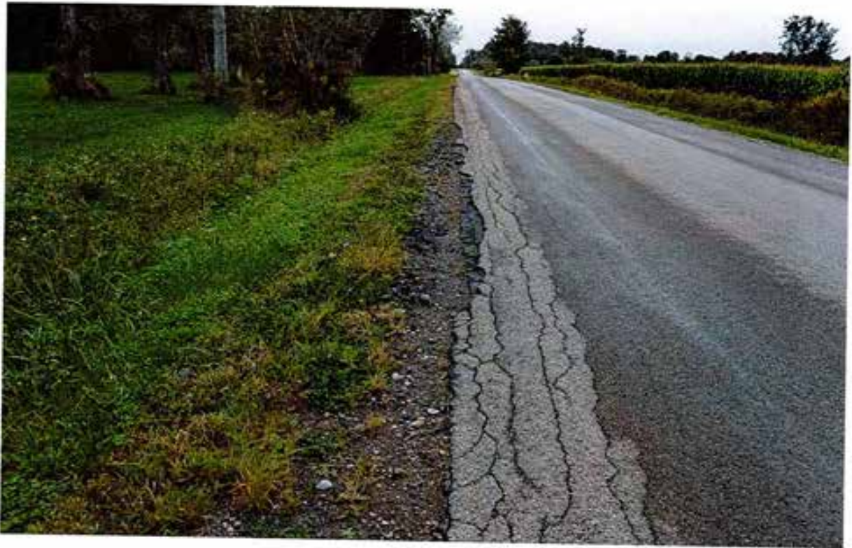
Brown Schoolhouse Road East shoulder deterioration South of 11748
