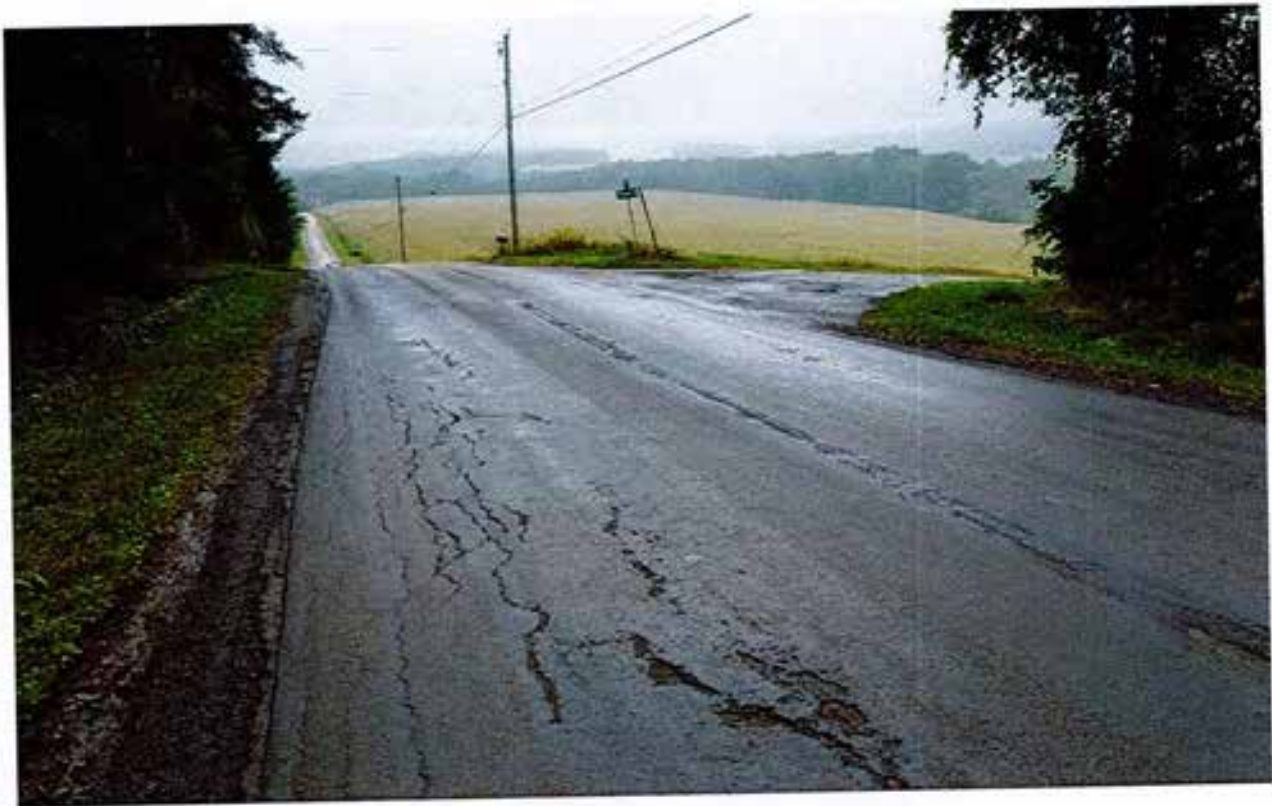
Galen Hill Road intersection with Phillippi Rd lane deterioration
