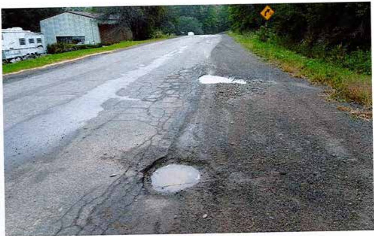
Osmun Rd Edge and shoulder deterioration near Zimmer
