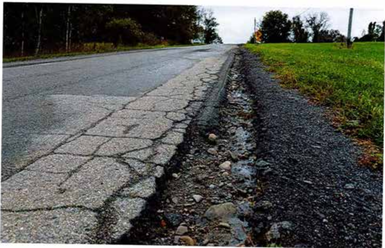
Hughes Road edge and shoulder deterioration on North and South sides East of 951
