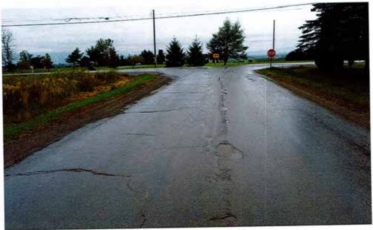
Lane deterioration North Rd near intersection with Bray Rd
