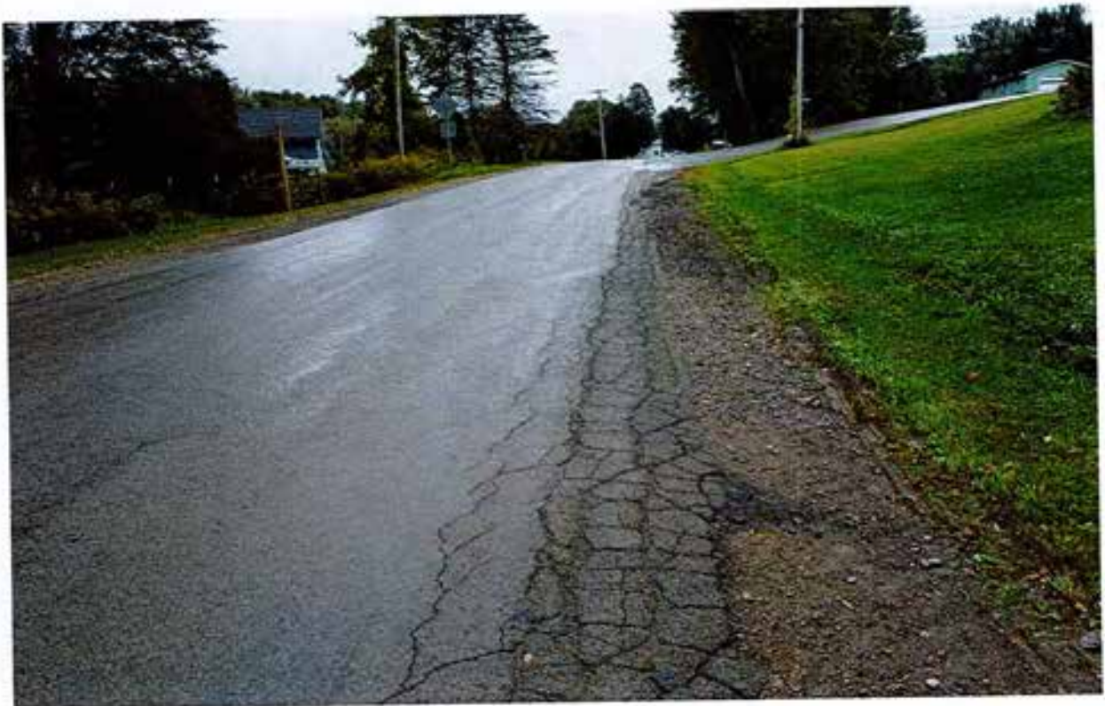
Eagle Street East edge deterioration near Hughes
