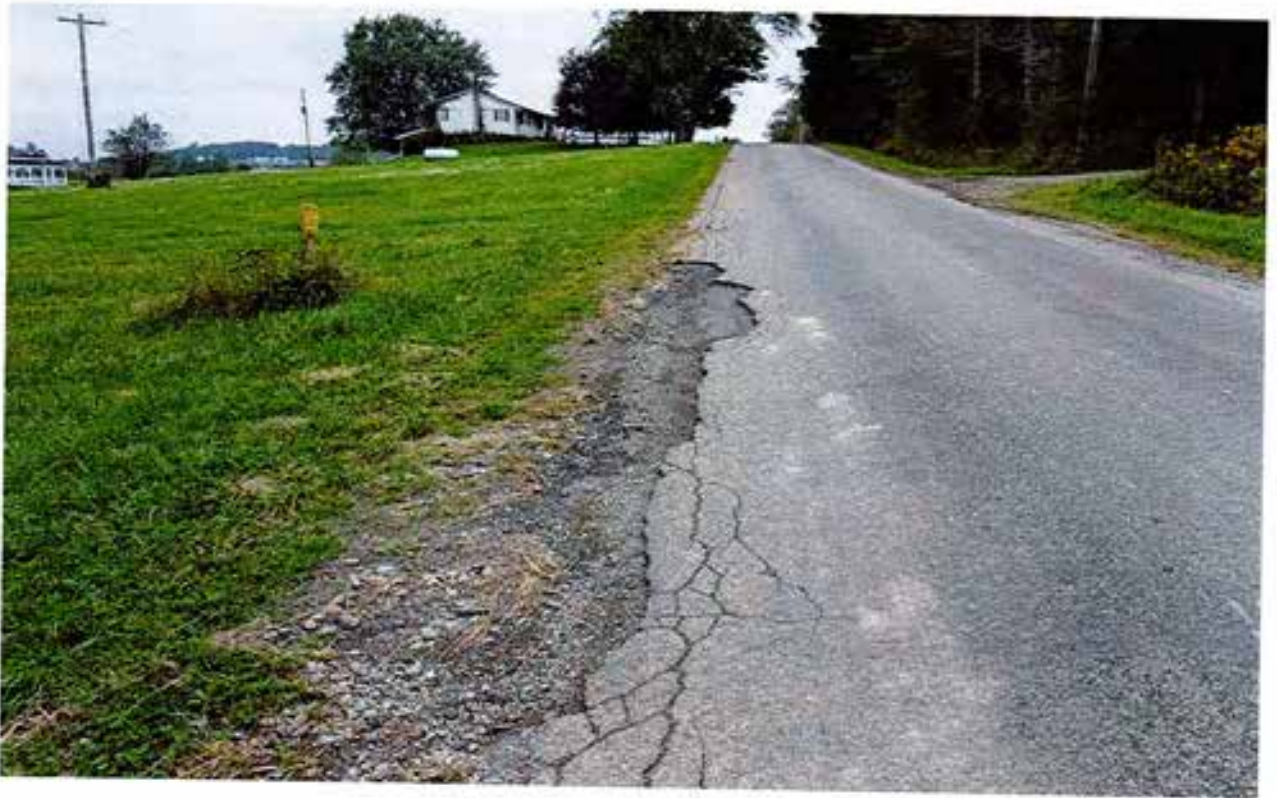
Sandbank Rd West lane and edge deterioration South of 10317
