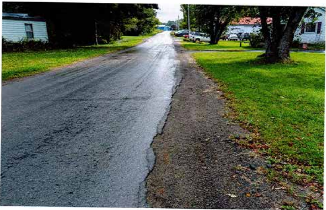
Eagle Street lane and edge deterioration near 1253
