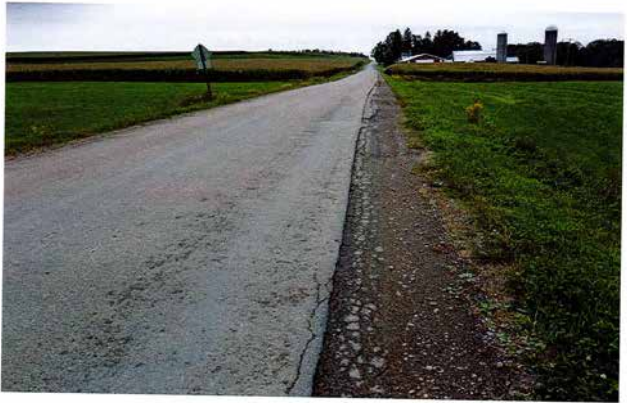
Brown Schoolhouse Road West shoulder deterioration from 11214 to 11123
