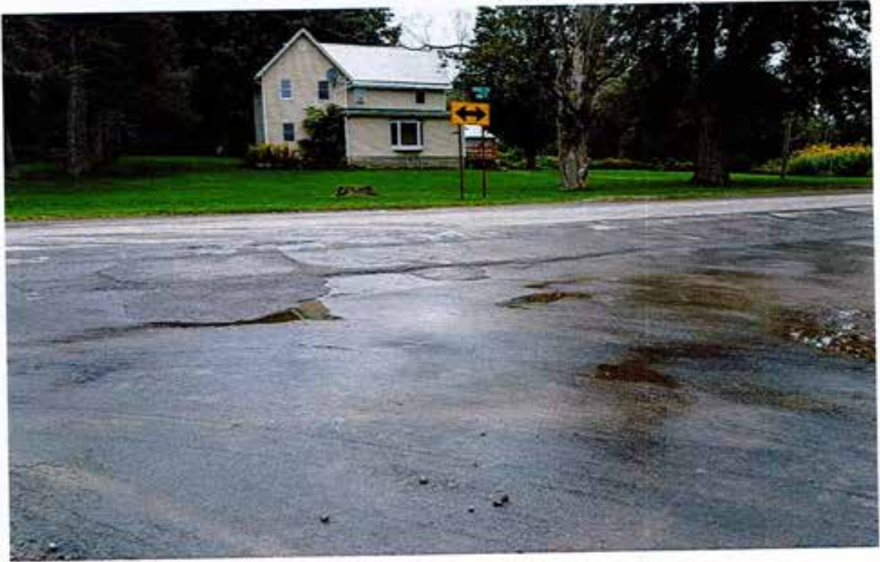
Bray Road lane deterioration near intersection with Eagle St
